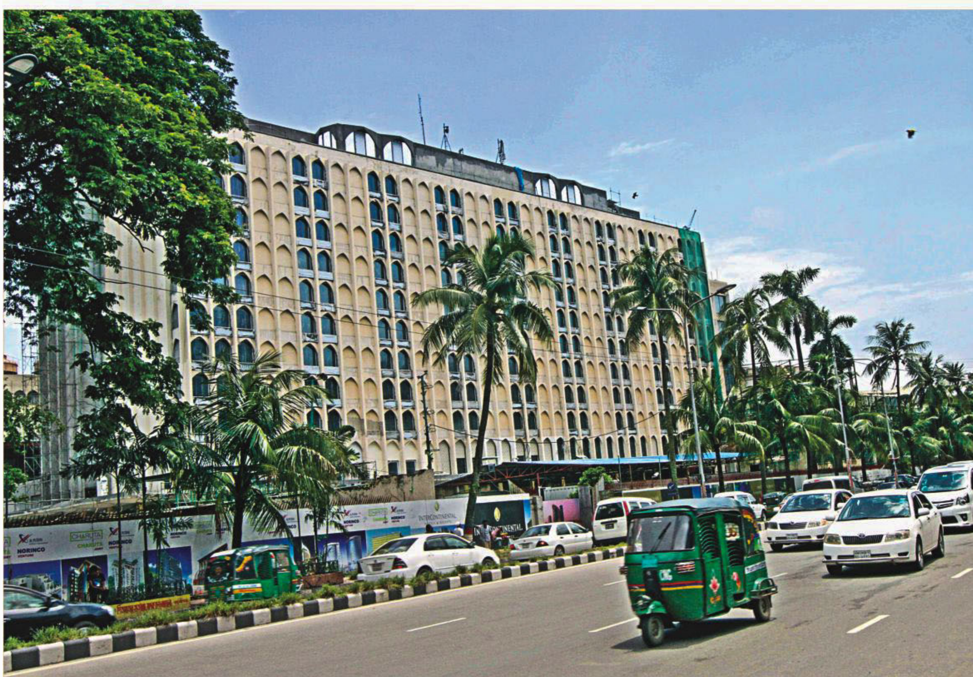
The renovation work of Ruposhi Bangla Hotel, formerly known as Sheraton Hotel, is underway. The re-opening of the hotel is likely to be delayed by several more months due to some complexities over its designs. The photo was taken recently.
