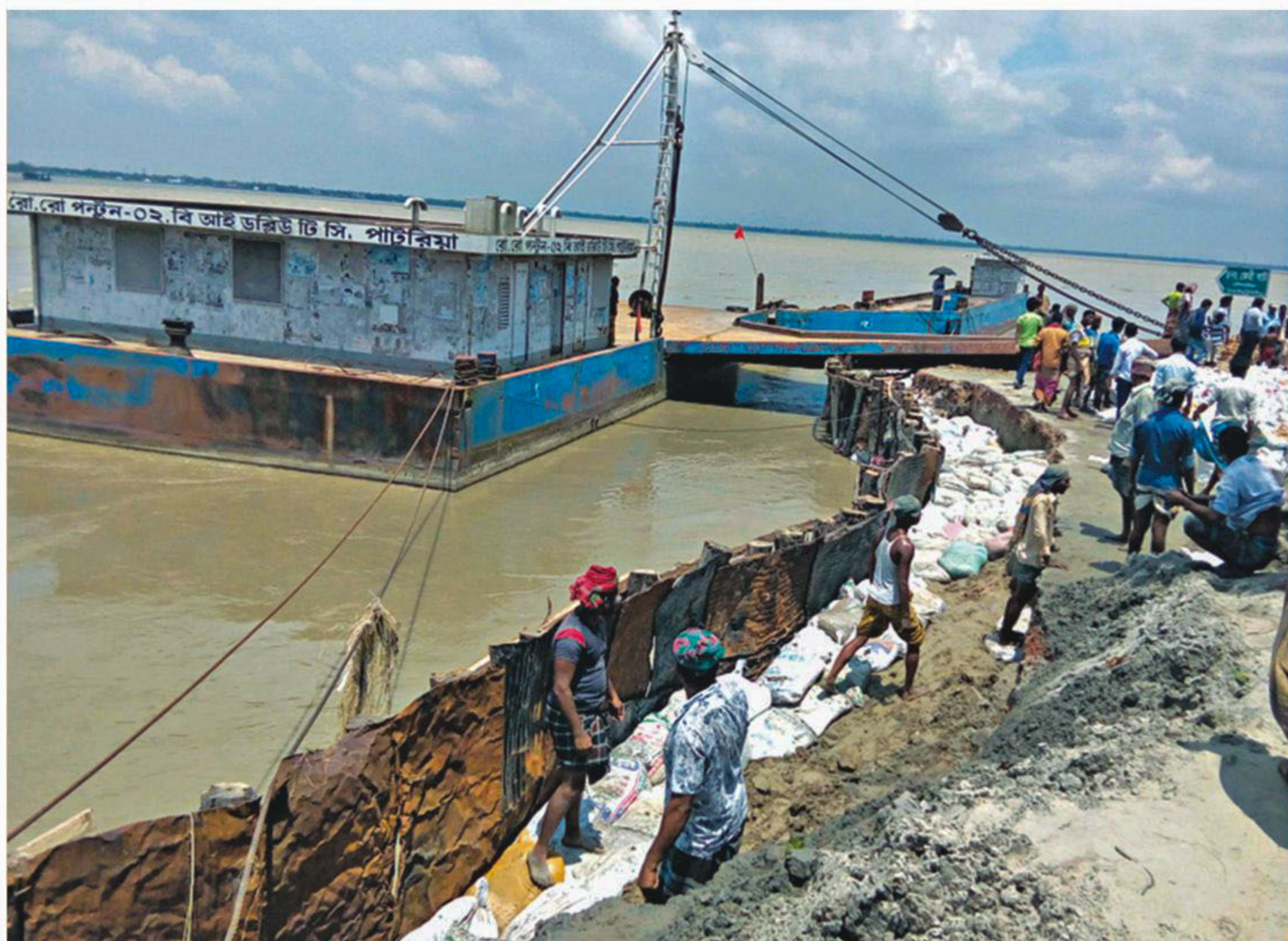
Labourers repair the approach road to the Landing Station-4 at Daulatdia ferry terminal in Rajbari by dumping sand bags. Ferry movement on Paturia-Daulatdia river route was suspended on Sunday, as the mighty Padma washed away three of the four landing stations at the terminal. The photo was taken yesterday.
