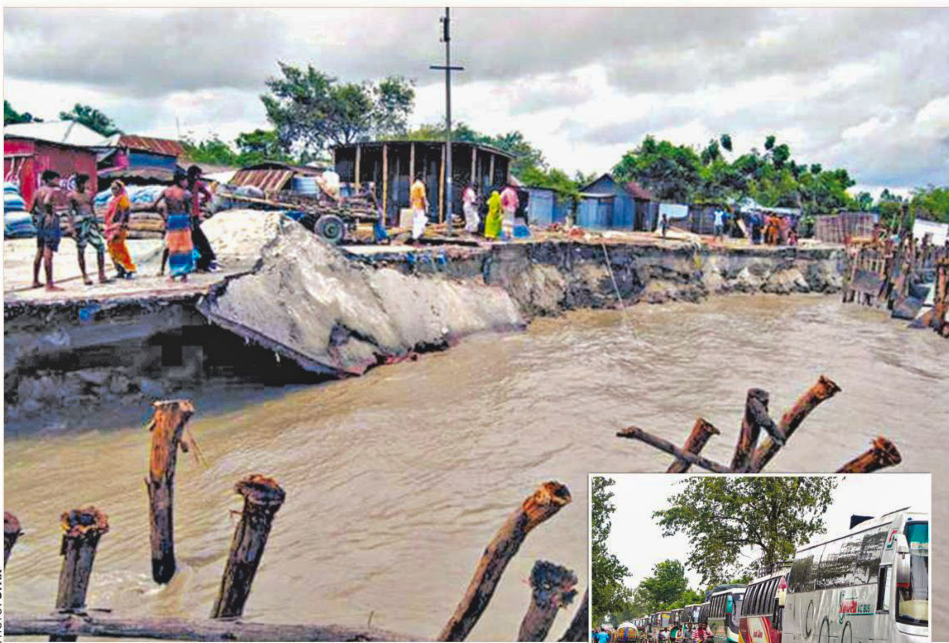
The Padma river devoured Landing Station-2 of Daulatdia ferry terminal in Rajbari on Saturday. It has led to traffic snarl-up on the approach road to the terminal, inset. The photos were taken yesterday.
