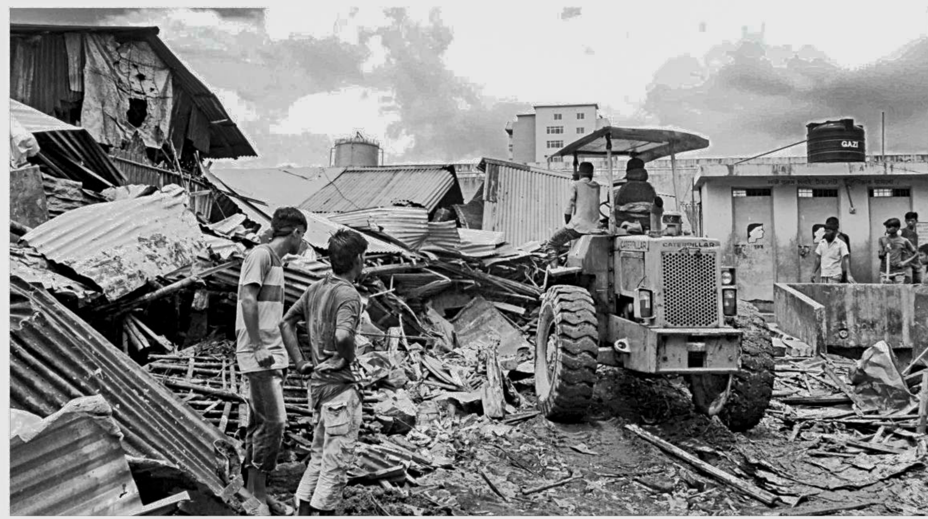
The Bangladesh Railway authorities demolishing illegal tin-roofed houses in the railway station land in the port city yesterday. Around 200 such houses and structures were demolished during the eviction drive assisted by Chittagong Metropolitan Police.
