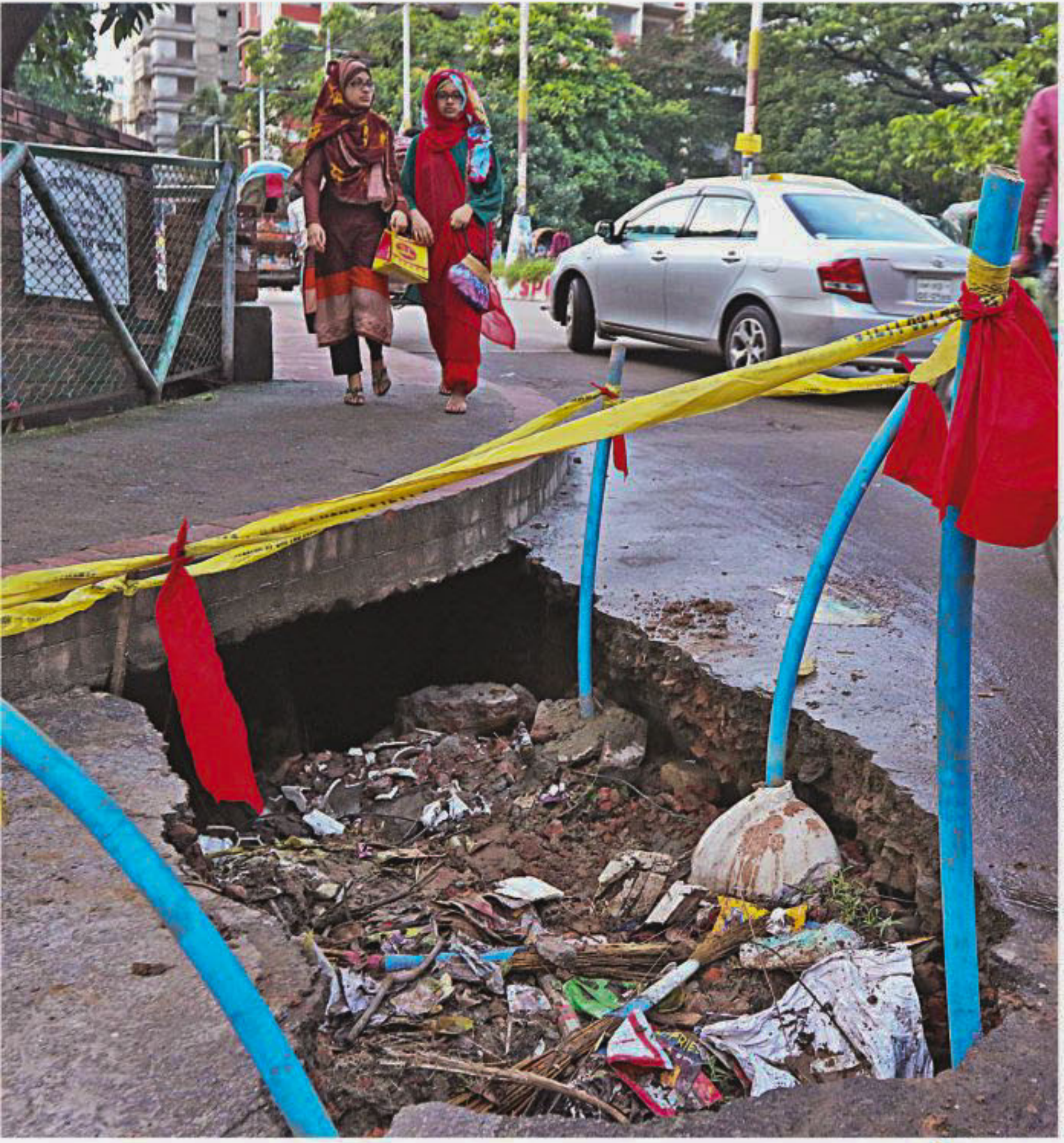
Though alerting pedestrians with barricade tape on poles, this dug up portion of the road on Dhanmondi 32 in the capital has left a hole, posing a risk of the footpath above to cave in and cause injuries. The photo was taken yesterday.
