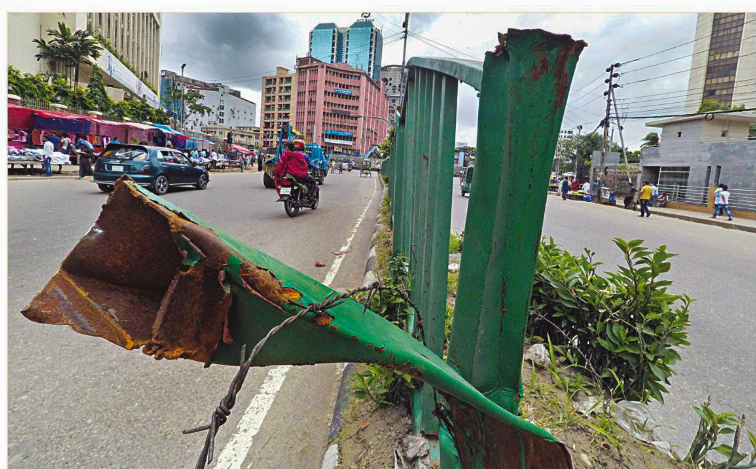
A part of the metal structure dividing the road in Shapla Chatter area of Motijheel in Dhaka has remained bent for a month, putting vehicles at risk of being hit against it any time. The photo was taken on Friday.
