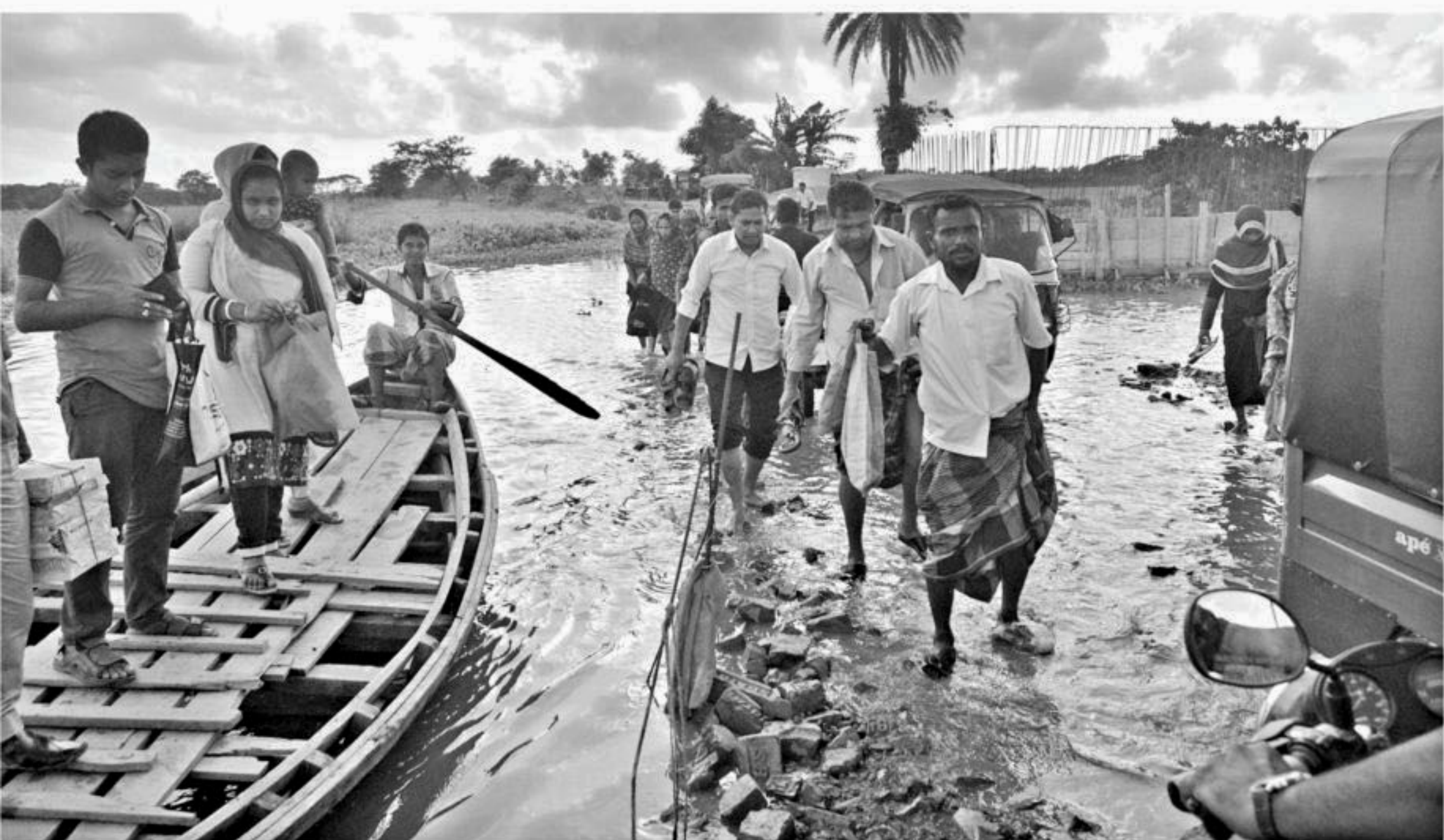
PHOTO: STAR The bypass, made to ease communication during bridge construction on Chankhar canal in Lohalia union of Patuakhali, has become synonymous with sufferings as inadequate work was done for the arrangement.
