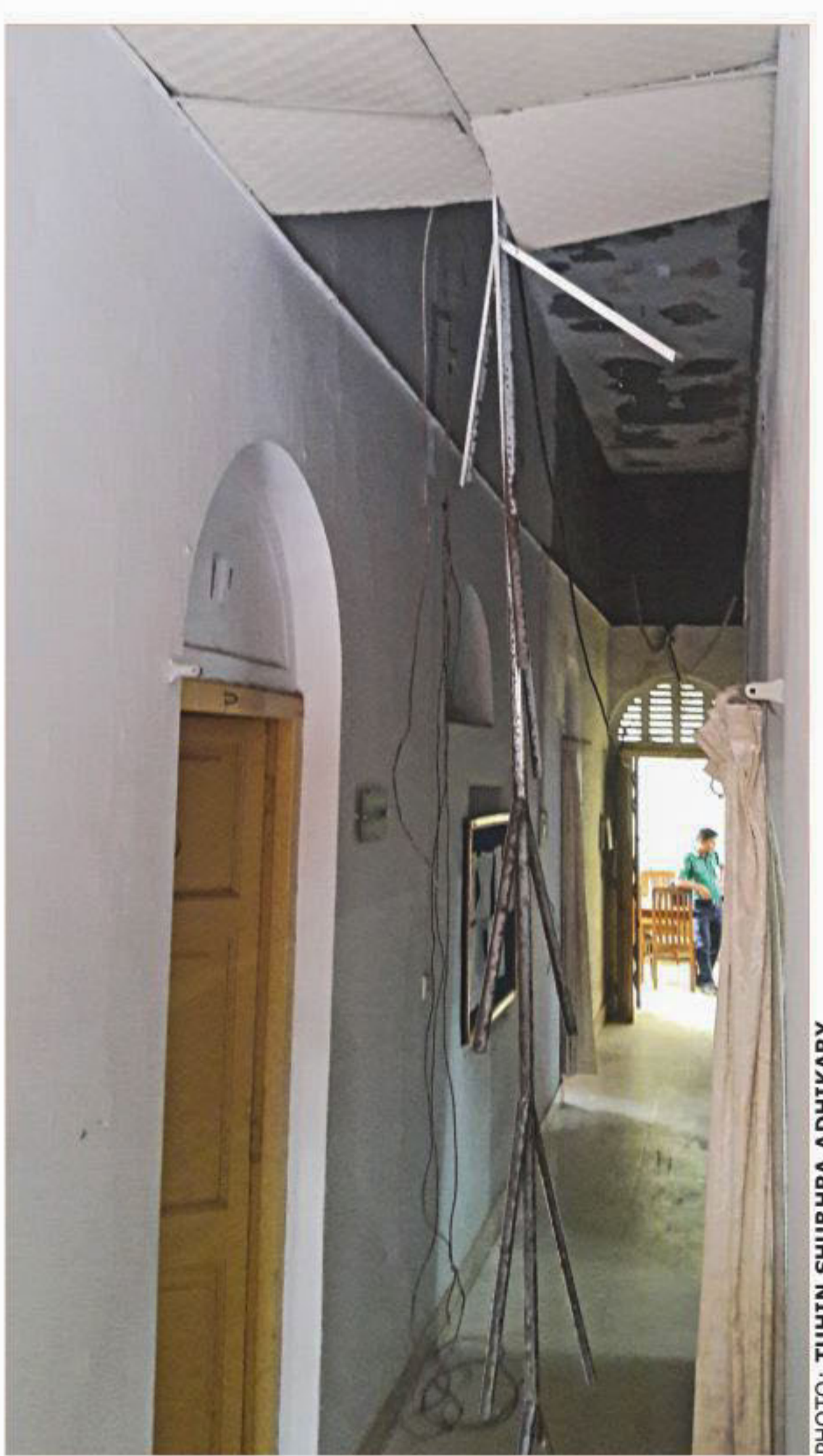
A portion of the ceiling of the old High Court building (west block) missing the false ceiling, which fell down yesterday morning, raising concerns among the prosecutors, whose office is situated there.
