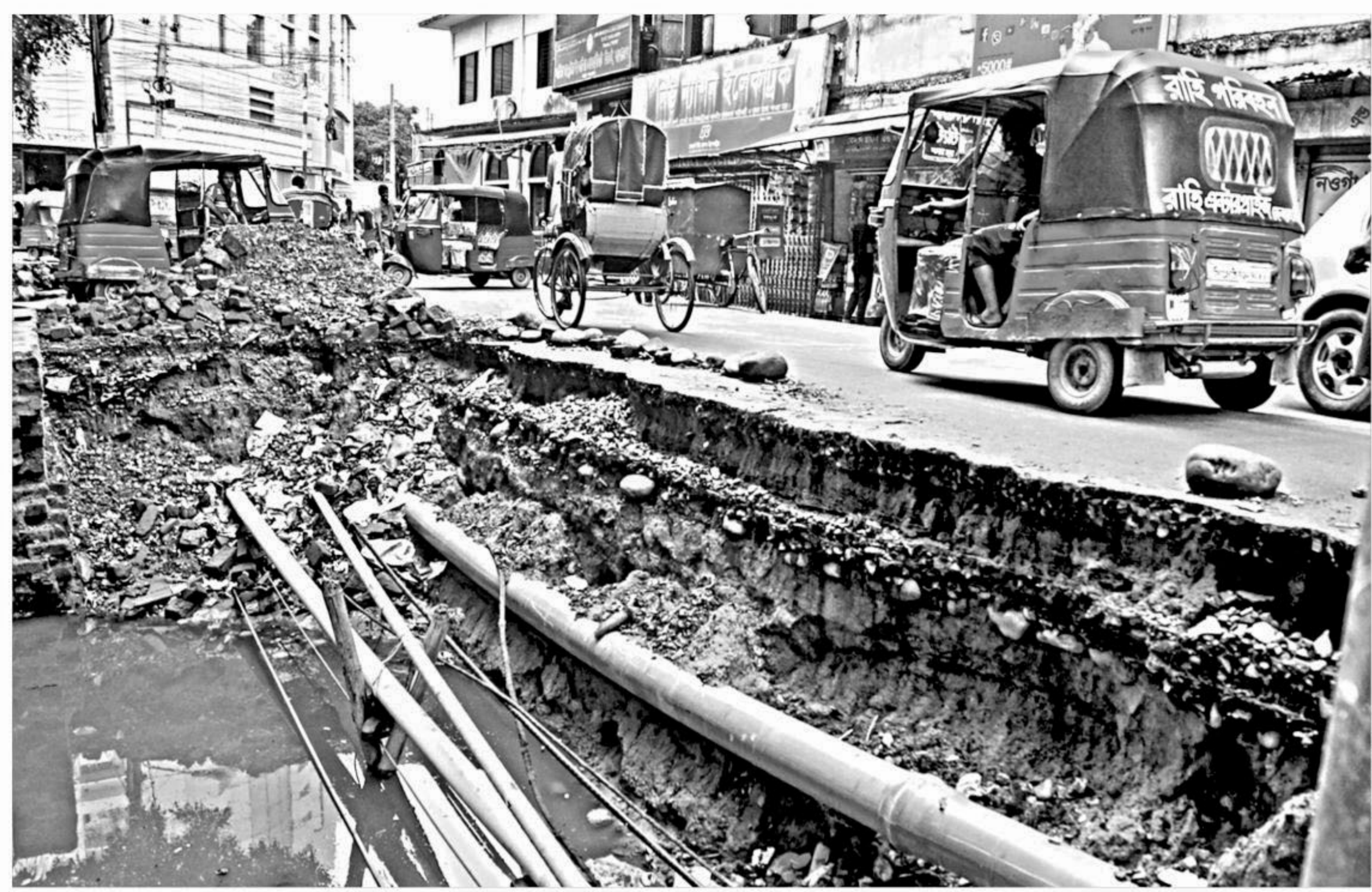
A half of the road in Sylhet city's Sobhanighat has remained dug up for more than a month, putting the vehicles and pedestrians at risk of falling into the ditch any moment. The city corporation has started digging the road for drainage and water pipeline works. The local ward councillor said the work would restart soon after the contractors entrusted with it get back from leave. The photo was taken on Monday.
