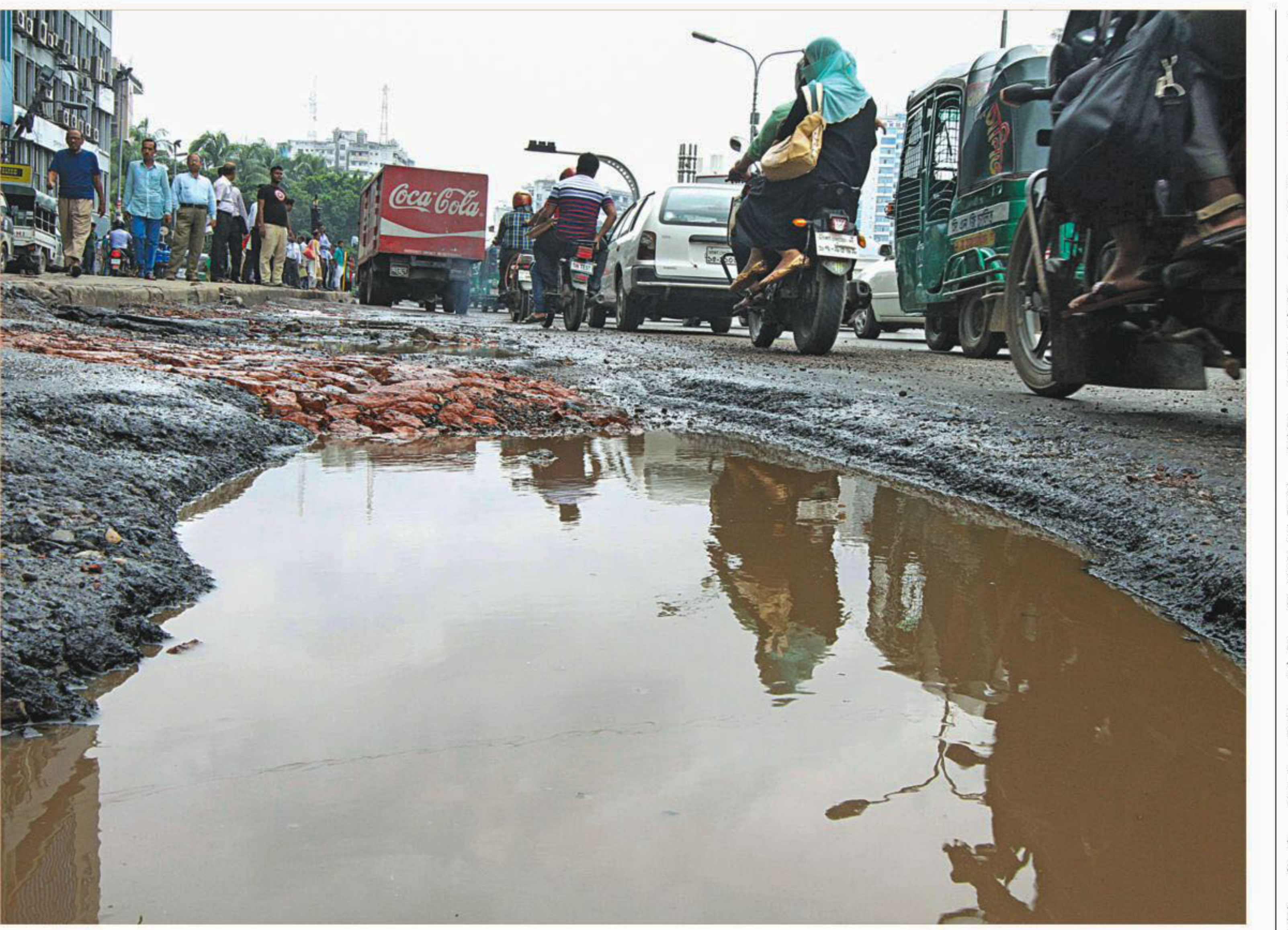
Even though the road is known as VIP road, these potholes veiled under the murky stagnant water were created just because of a few days' rainfall, an eventual result of poor construction work and lack of maintenance.
