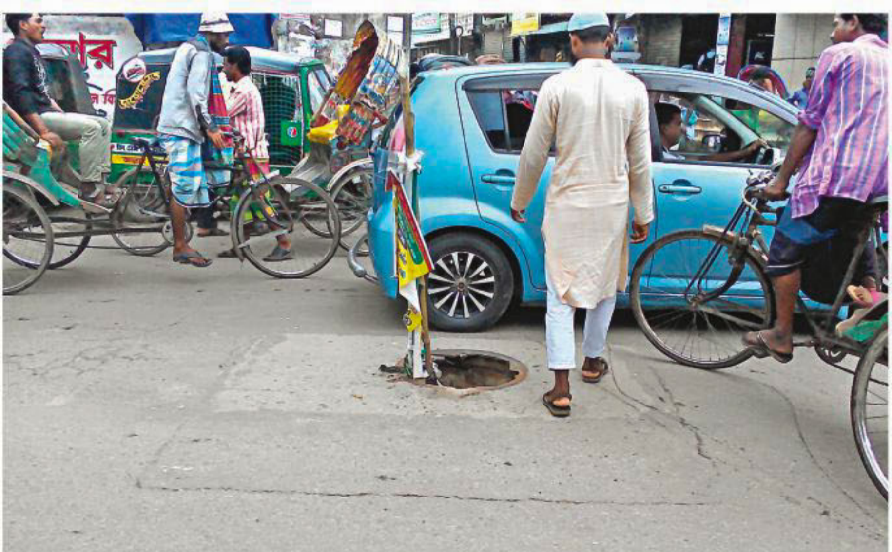
A manhole without its lid for the last one month in Katherpool area of the capital's Sutrapur yesterday. As the Dhaka South City Corporation (DSCC) "did not notice" it, local people have put a bamboo pole there to warn people against dangers.
