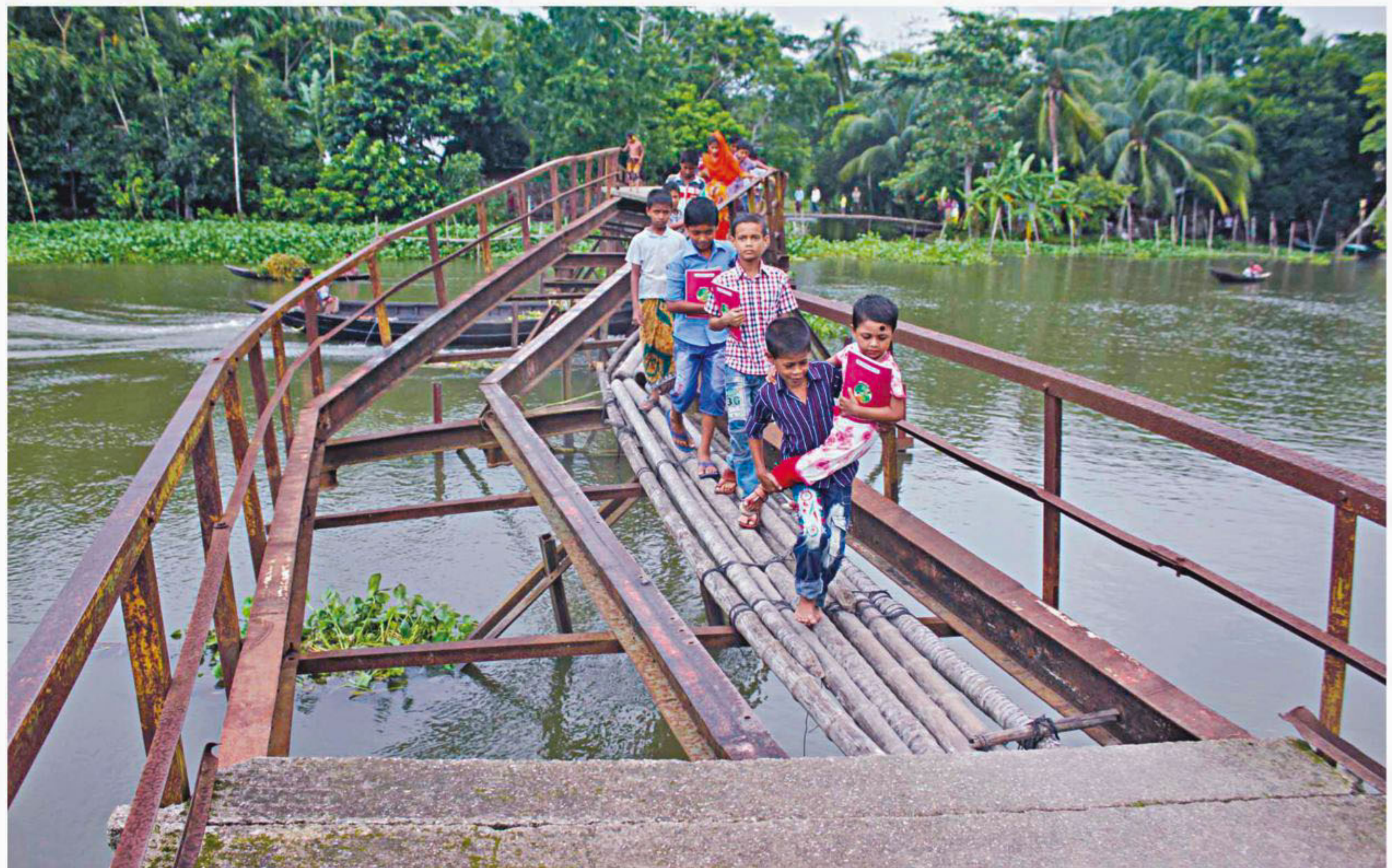
Children crossing a damaged bridge over Bisharkandi canal in Barisal's Banaripara recently. Locals are suffering as the bridge has been lying broken for around four years.
