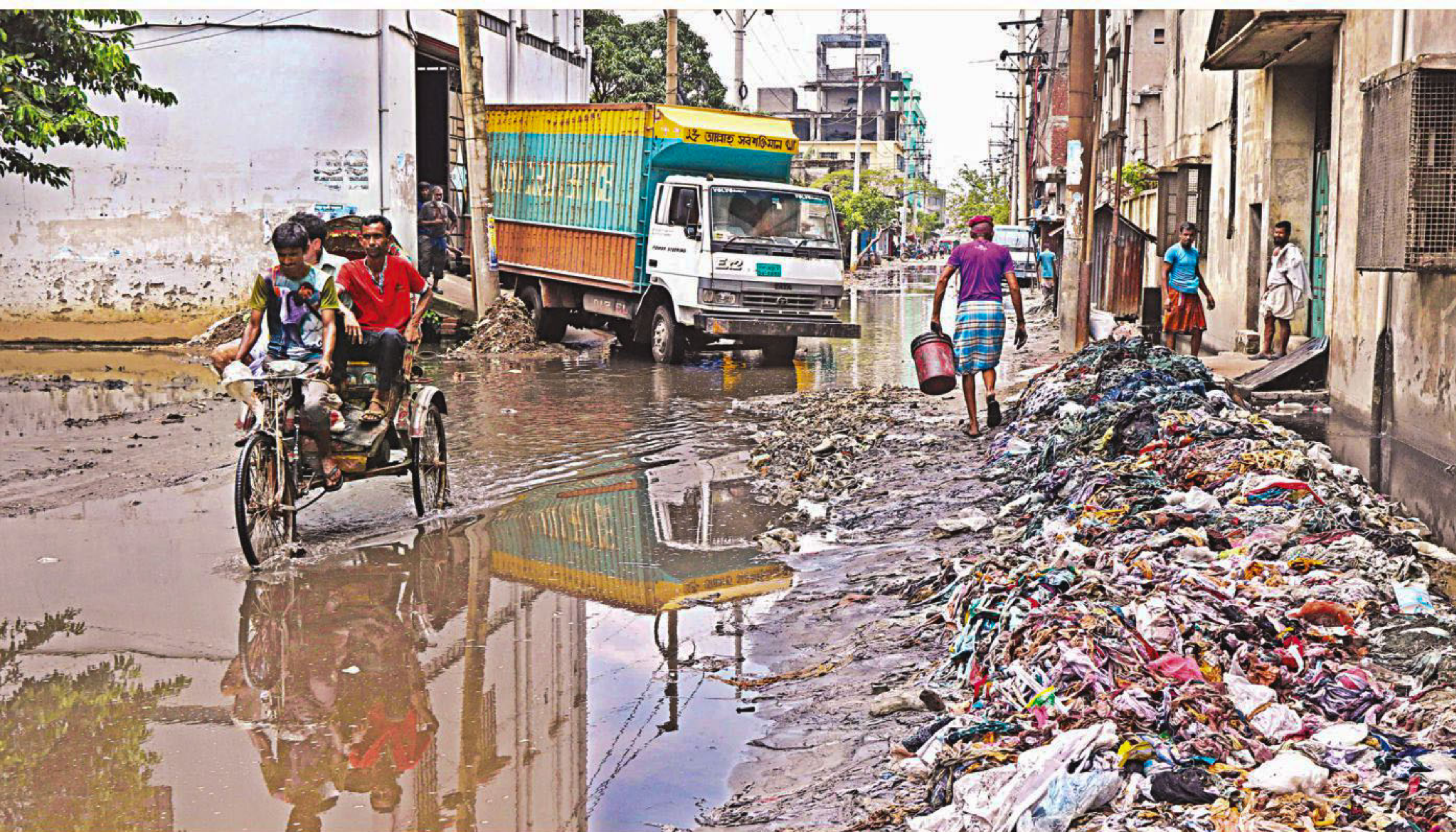
Renovation has long eluded this nearly inoperable road in the capital's DIT industrial area, where some 200 big and small factories are located. Some factory staff said the 13 roads in the area had been in a dilapidated condition for the last five years. The photo was taken yesterday.
