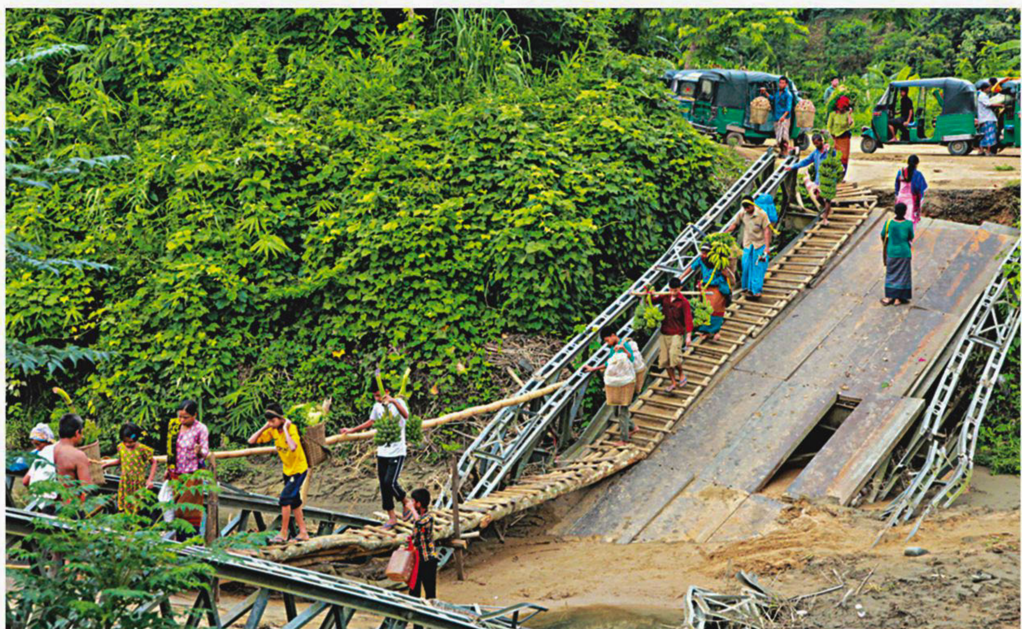
Farmers use a makeshift bamboo structure, built on this collapsed Bailey bridge, to carry their produce for sale in Kawkhali upazila of Rangamati recently. Road communications between Rangamati and Bandarban remain snapped for the last three months since the bridge collapsed. The authorities concerned are yet to take any step to repair it.
