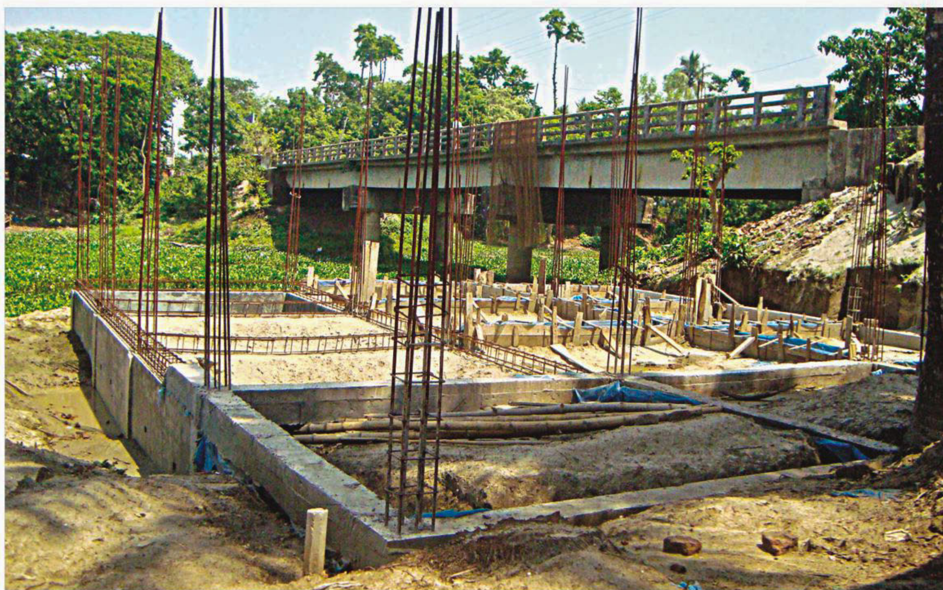
Construction of this large building on the land of the Kobadak beside Alampur Bridge in Moheshpur upazila under Jhenidah district further squeezes the already decaying river.
