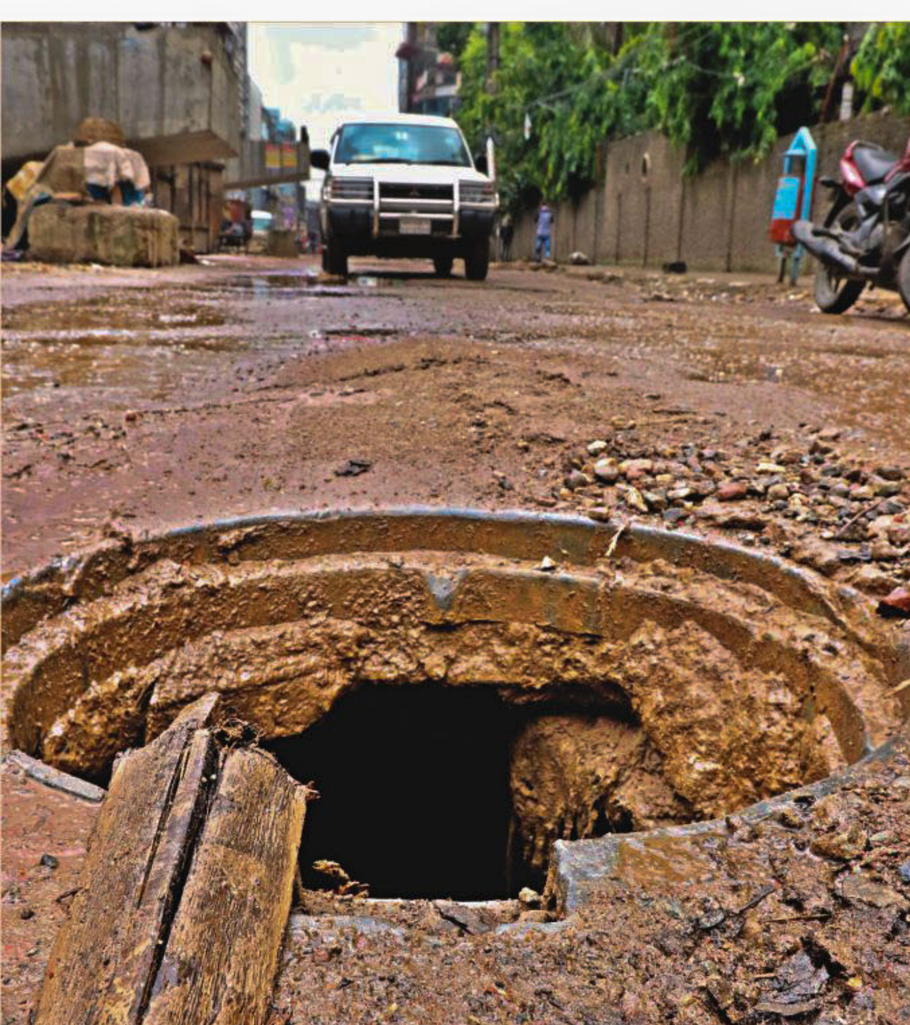
A sewer opening sans the lid right in front of the Rajarbagh Police Lines in the capital, posing the risk of an accident anytime. The photo was taken yesterday noon.
