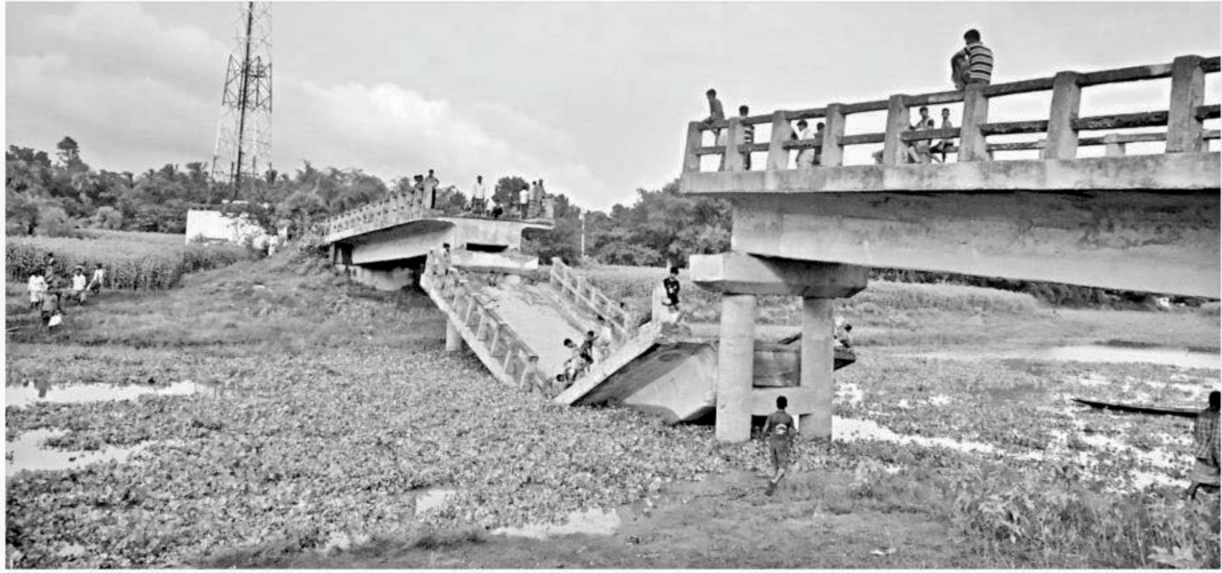
A bridge over the River Sanchi under Jhenidah Sadar upazila collapsed in Jhenidah on June 6. PHOTO: AZIBOR RAHMAN
