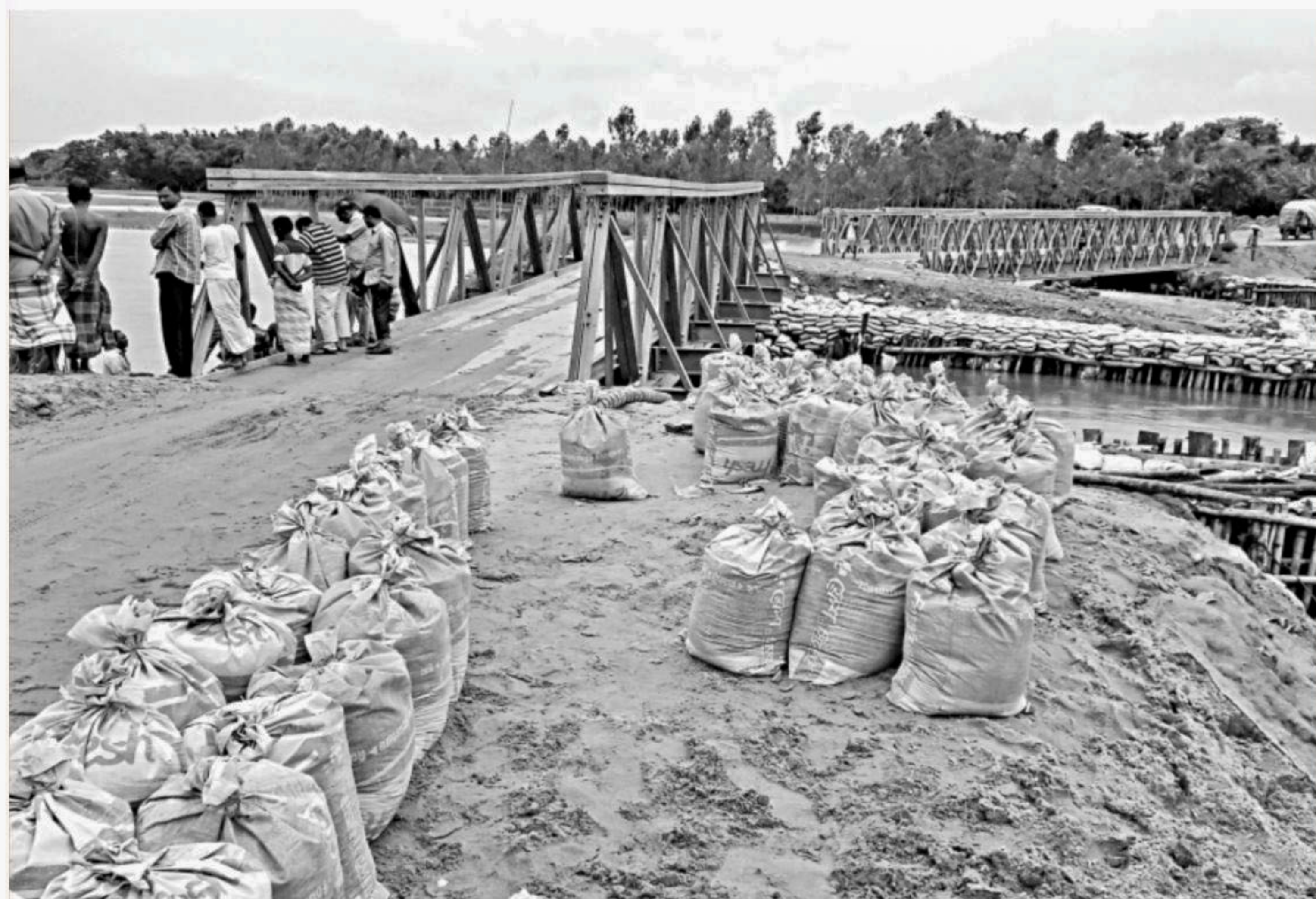
Sacks full of sand are being dumped in the Swarnamoti River on Lalmonirhat-Burimari highway at Sarpukur village under Aditmari upazila to protect the vulnerable bailey bridge as it is in danger of collapsing due to surge of water and movement of heavily loaded trucks. PHOTO: STAR
