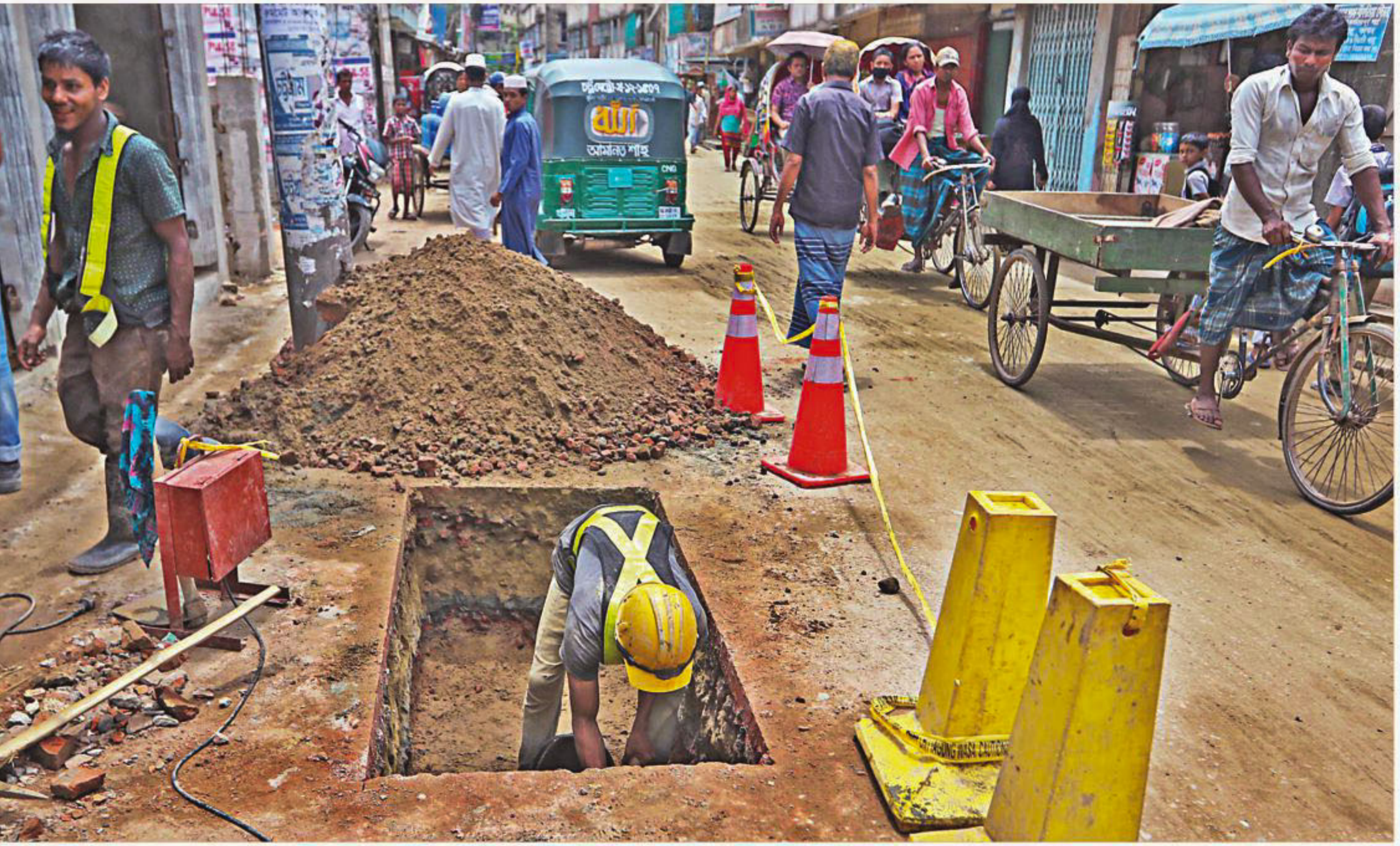
The Water Supply and Sewerage Authority (Wasa) digging a pit on the newly paved KB Aman Ali road in Chittagong city recently, to install sewers. Due to a lack of coordination with the Chittagong City Corporation (CCC), which constructed the road, damage is being done to the street, prolonging public sufferings, causing traffic congestion, and leading to waste of public money. PHOTO: ANURUP KANTI DAS
