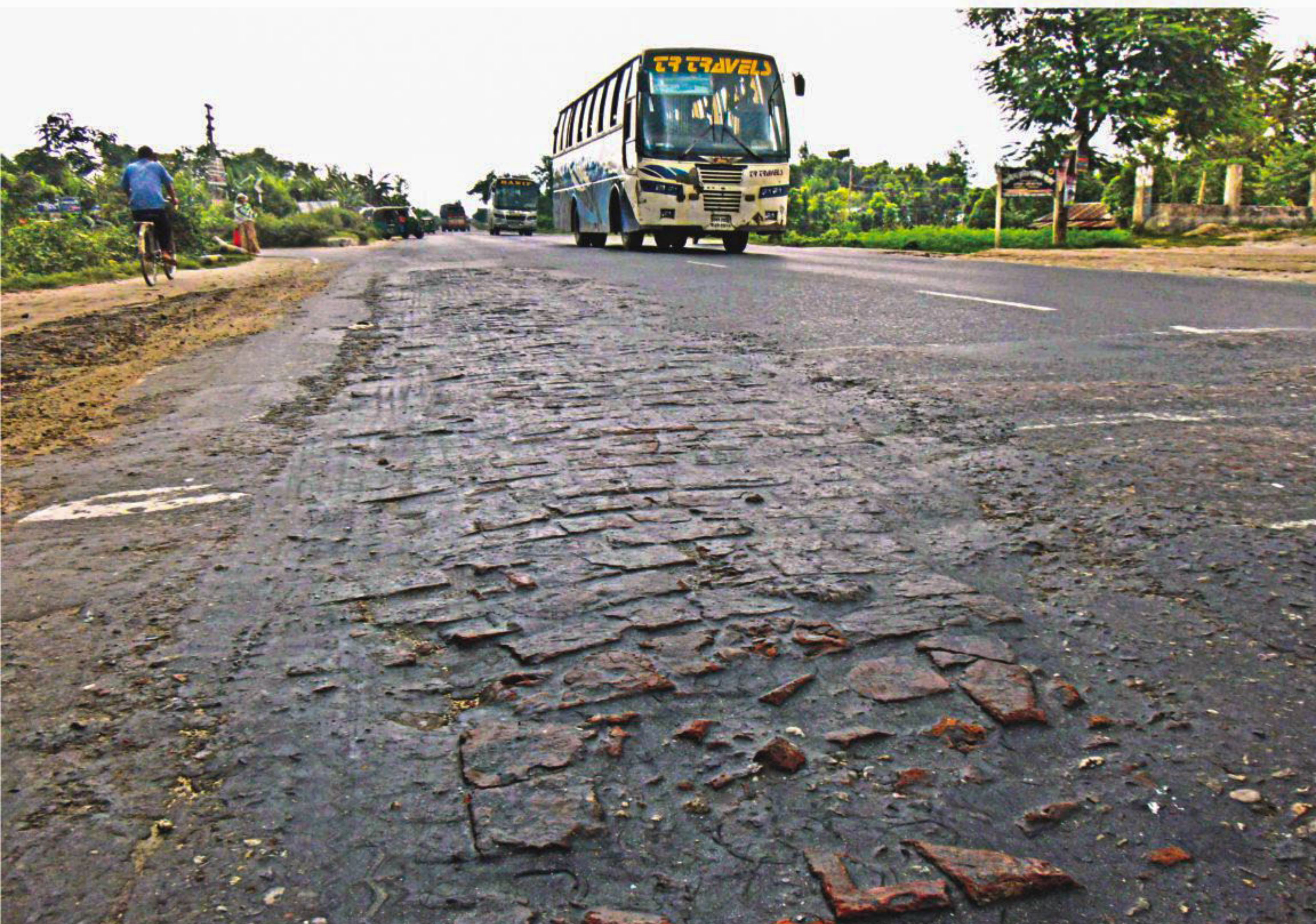
Large potholes in Dhaka-Tangail highway at Bhakurta of Tangail have been poorly patched up with bricks by the Roads and Highways Department ahead of Eid. Transport drivers and highway police said the road would be damaged even after a light rain.
