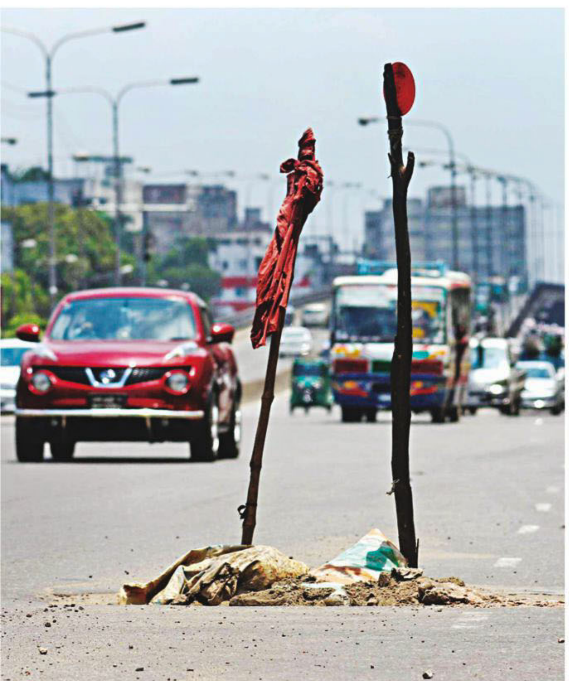
Sticks propped up on a manhole broken for long near the end of the Mohakhali flyover ramp, which lets vehicles head towards Chairmanbari, by nearby traders who claim some 10 accidents occurred there involving unsuspecting drivers. The photo was taken yesterday noon.
