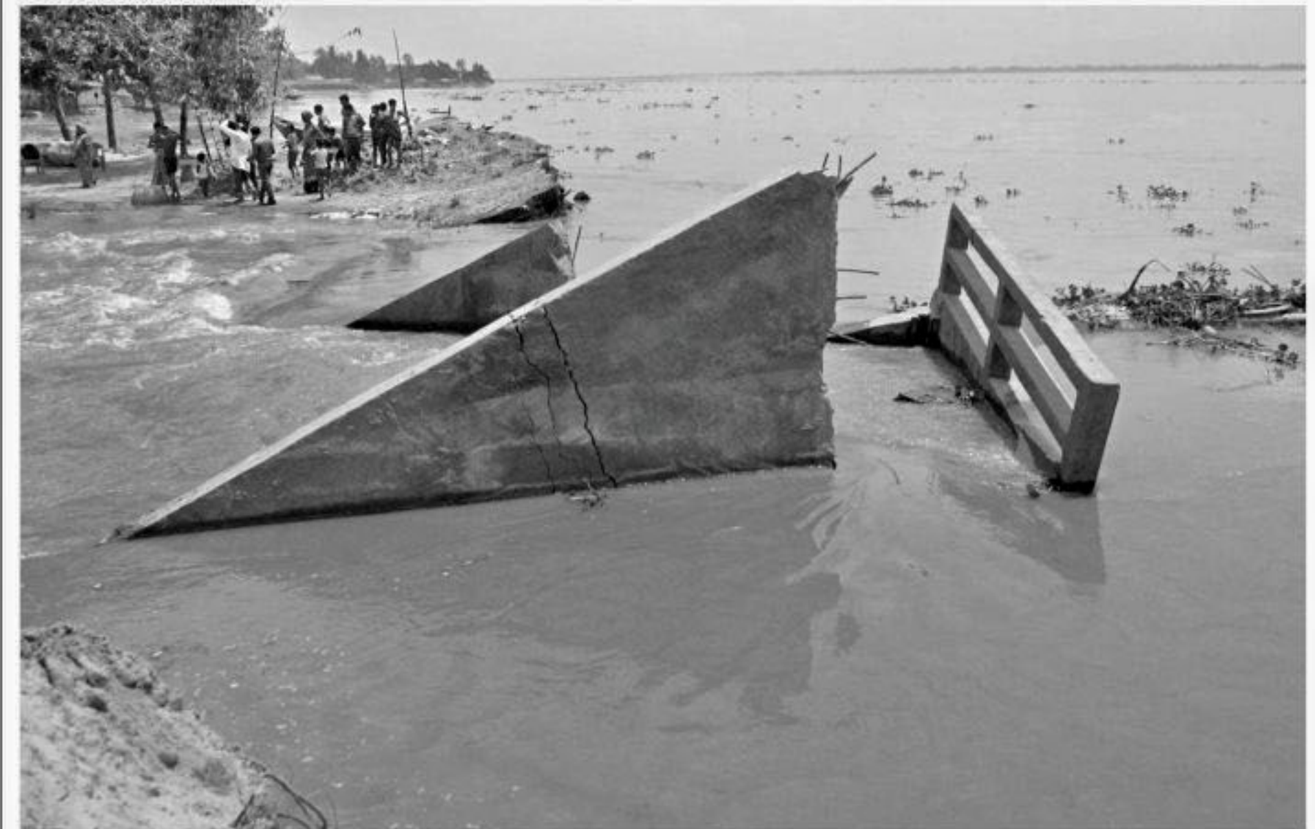
Around 20 villages got flooded as this sluice gate in Saghata upazila under Gaibandha district collapsed under the pressure of the swelling Jamuna River on Thursday.
