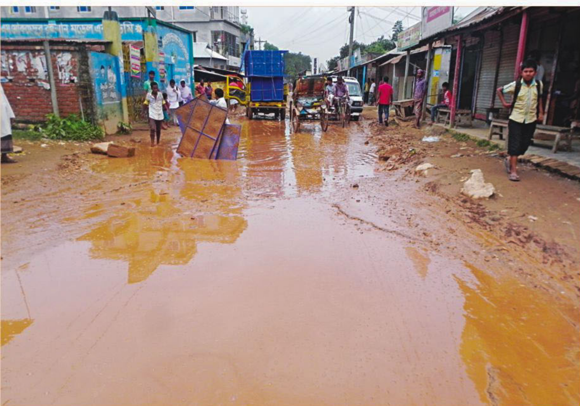
Vehicles struggle to move over Joina Bazar-Kaoraid road in Sreepur upazila of Gazipur as the waterlogged portion stretching half a kilometre of the road got completely damaged with the monsoon beginning this year. The photo was taken recently.
