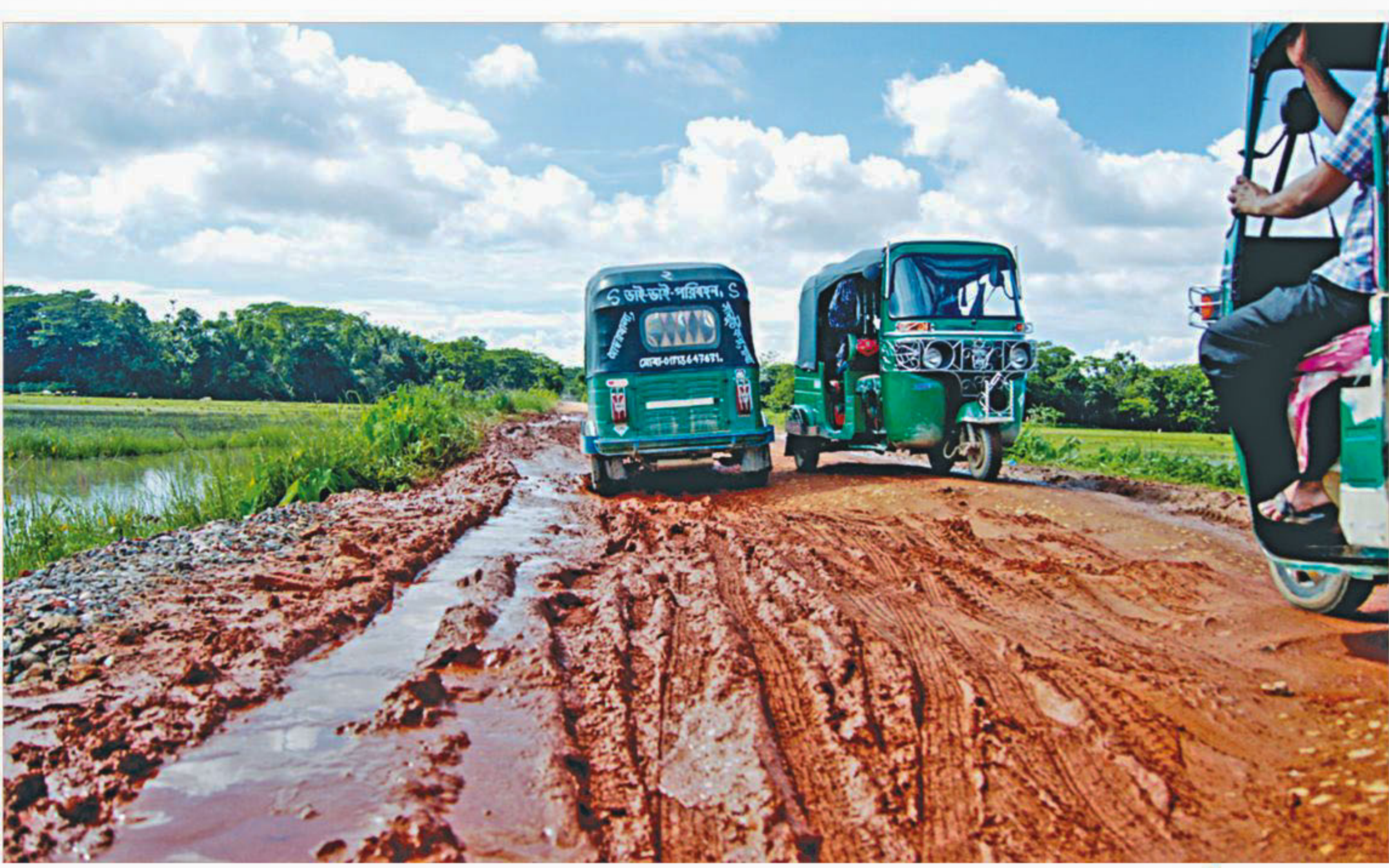
This road, connecting Shalutikkor-Sylhet-Shiberbazar, is slowly breaking down, unable to take the load of some 10,000 to 12,000 vehicles using it every day as an alternative to the one connecting Sylhet-Companyganj-Belaganj, which is in such a dilapidated state that only big wheelers can now ply on it. The photo was taken yesterday.
