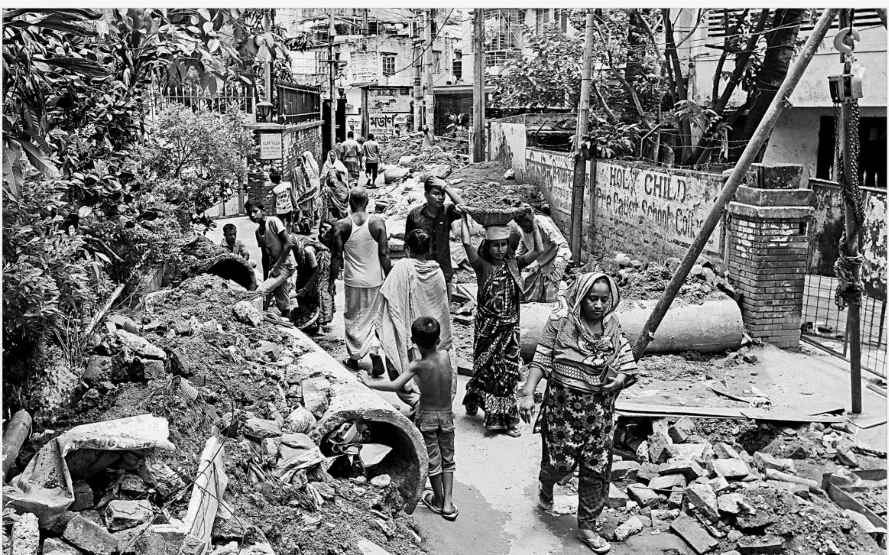
Pedestrians pass through this road which has been narrowed down as broken underground pipes have been kept there for its development works for around 18 days in Pearabagh of the capital's Moghbazar. The photo was taken yesterday.
