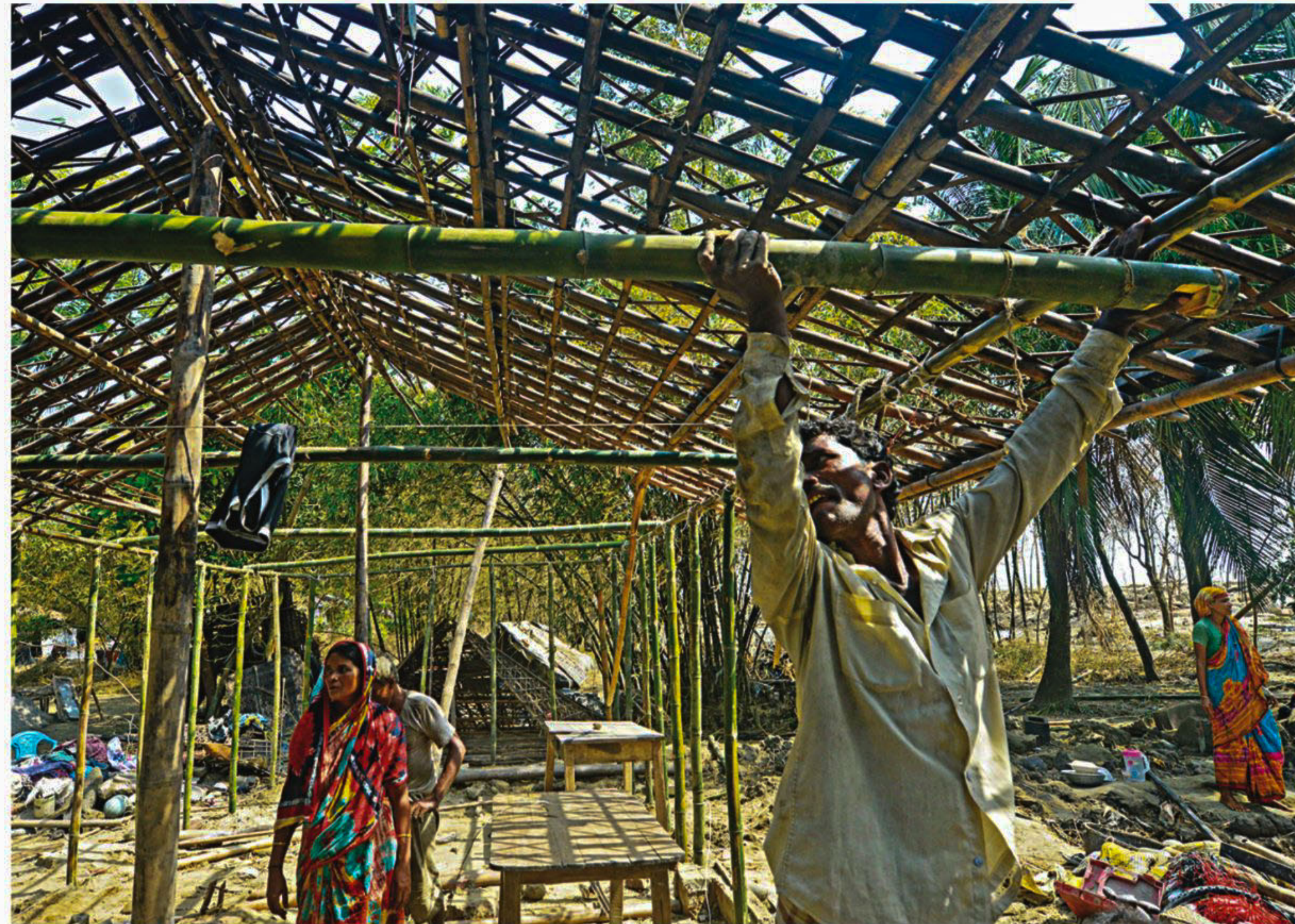
A family rebuilds their home. The homes are usually made of planks, bamboo and tin sheets which are cheap and easy to acquire. However, these materials are also the reason homes are non-resilient to storms and are at constant risk from cyclones. Kajir Para in Kutubdia is still in the process of rebuilding itself.
