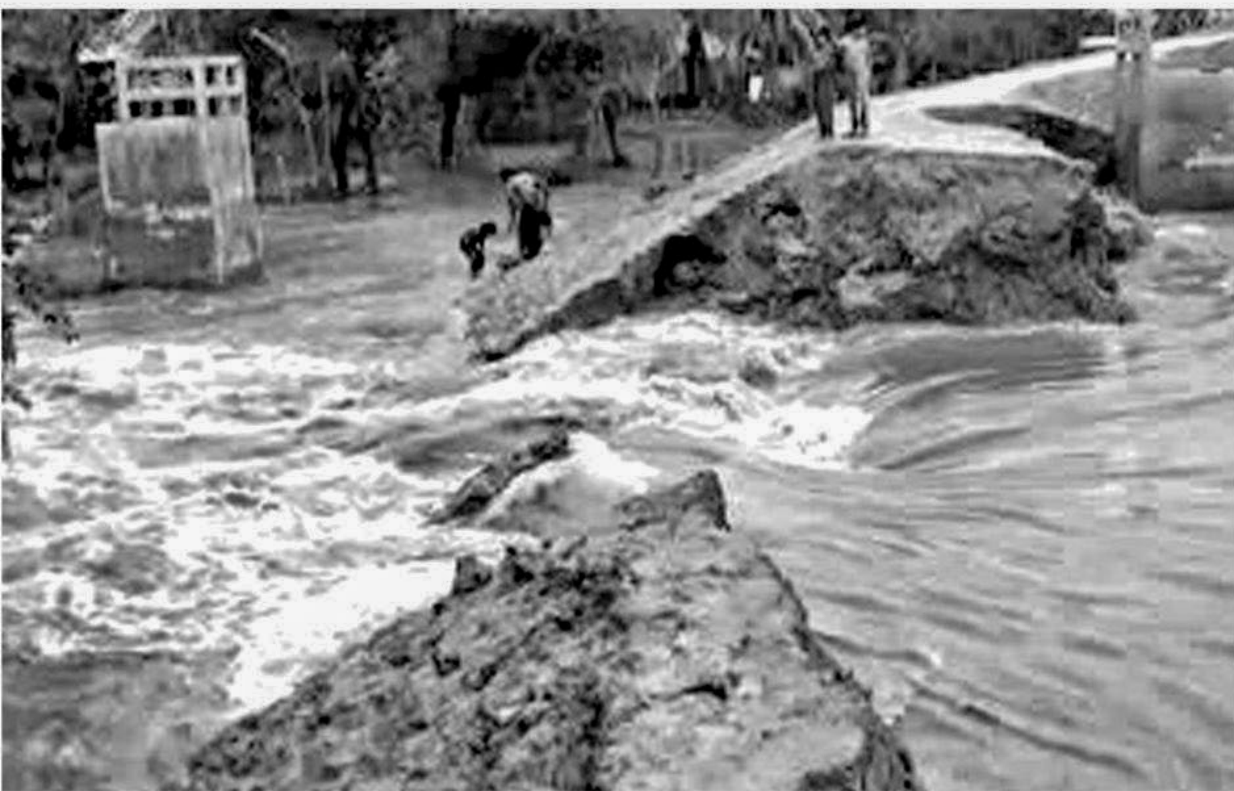
Breach in this embankment in Kalapara upazila under Patuakhali district has led to flooding of farmlands and fish enclosures in the area with saline water from tides.
