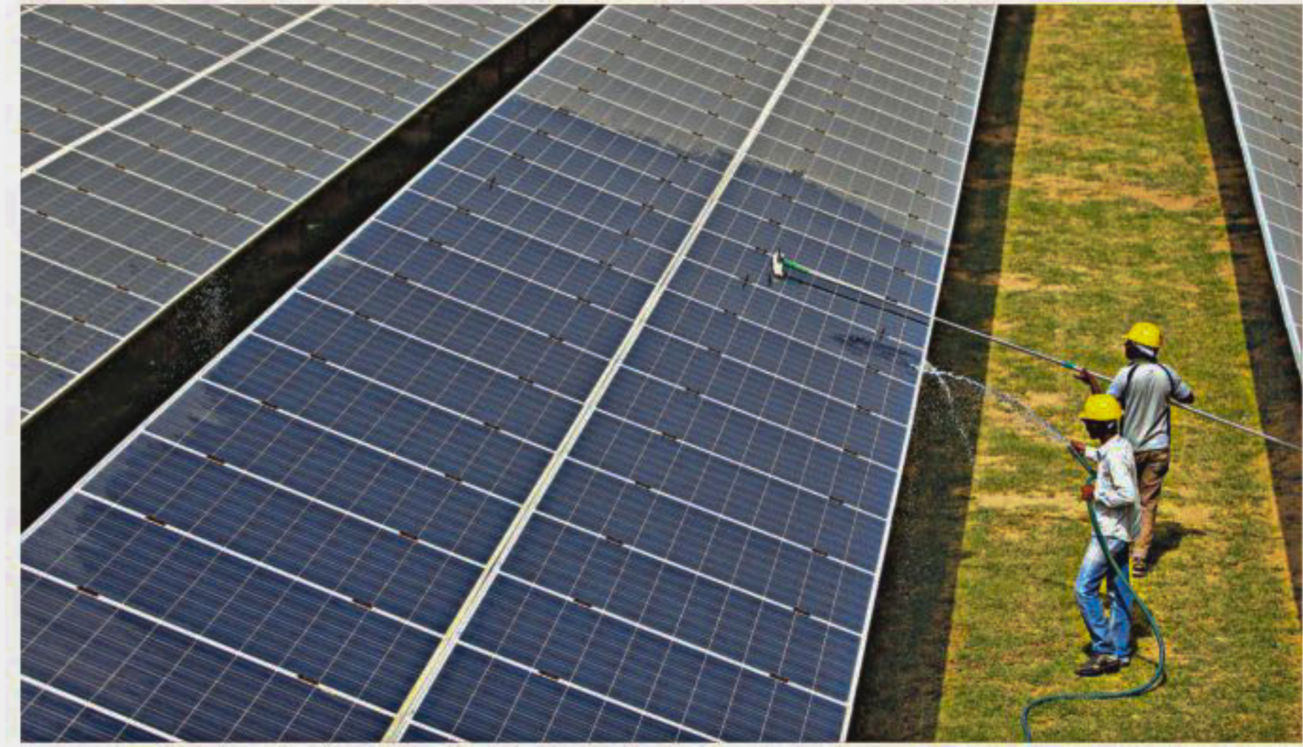
Workers clean photovoltaic panels inside a solar power plant in Gujarat, India.
