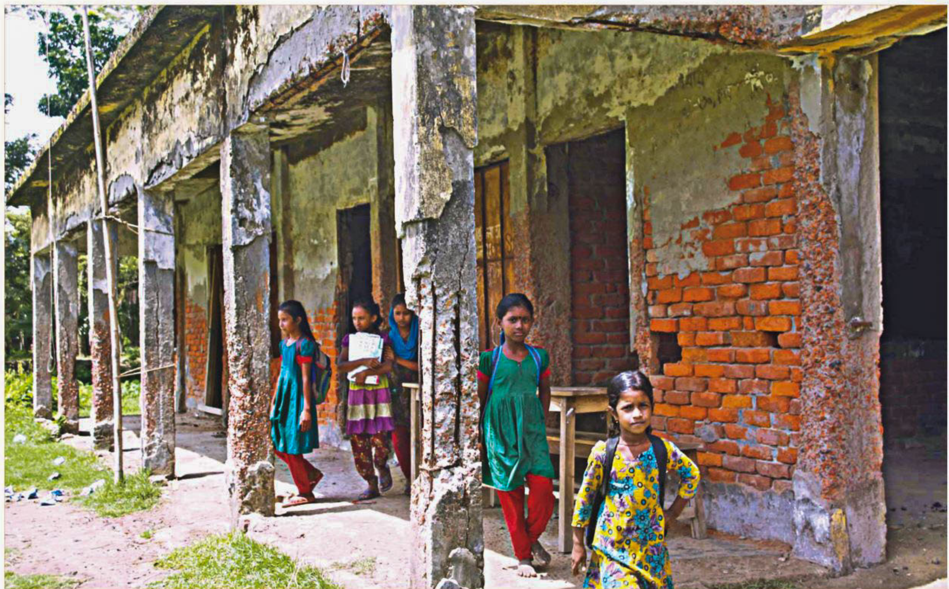
The dilapidated Dakkhin Kazir Howla Govt Primary School in Rangabali upazila of Patuakhali. Parents fear the building might collapse anytime due to lack of maintenance. The photo was taken recently.
