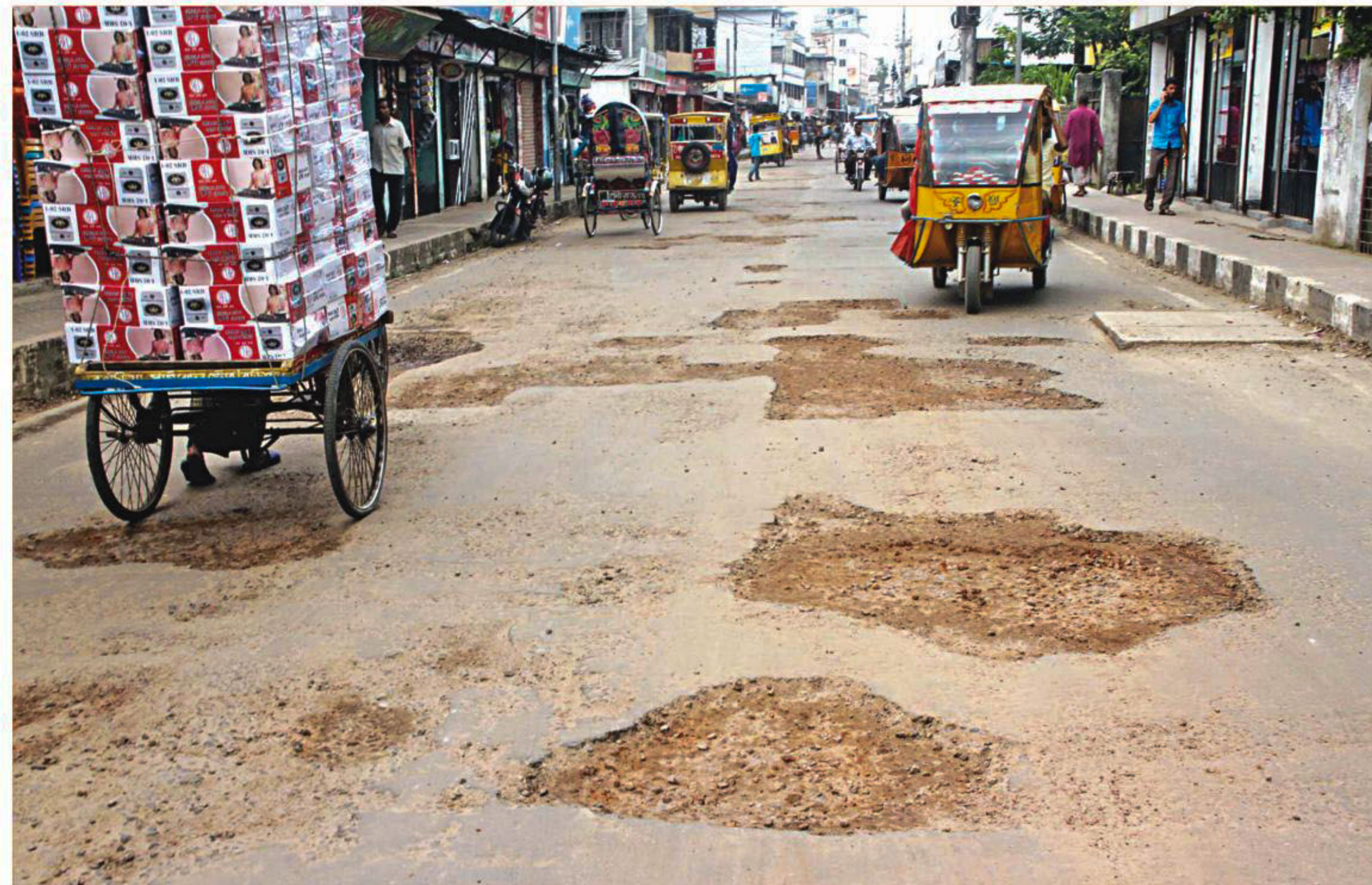
With cyclone Roanu and heavy rainfall severely damaging most of the roads in Barisal city, it has become a nightmare for the residents to take a ride on any mode of transport. The photo was taken recently in the city's Banglabazar Hospital Road area.
