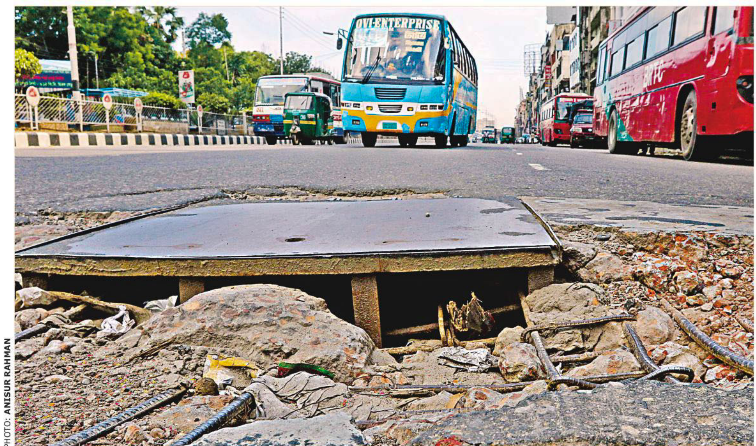
As asphalt around this underground utility cable pocket pulled out in the middle of Bir Uttam Ziaur Rahman Road, it has been left unprotected for quite a long time, which could cause a deadly traffic accident anytime. The photo was taken yesterday in Chairman Bari area of the capital.
