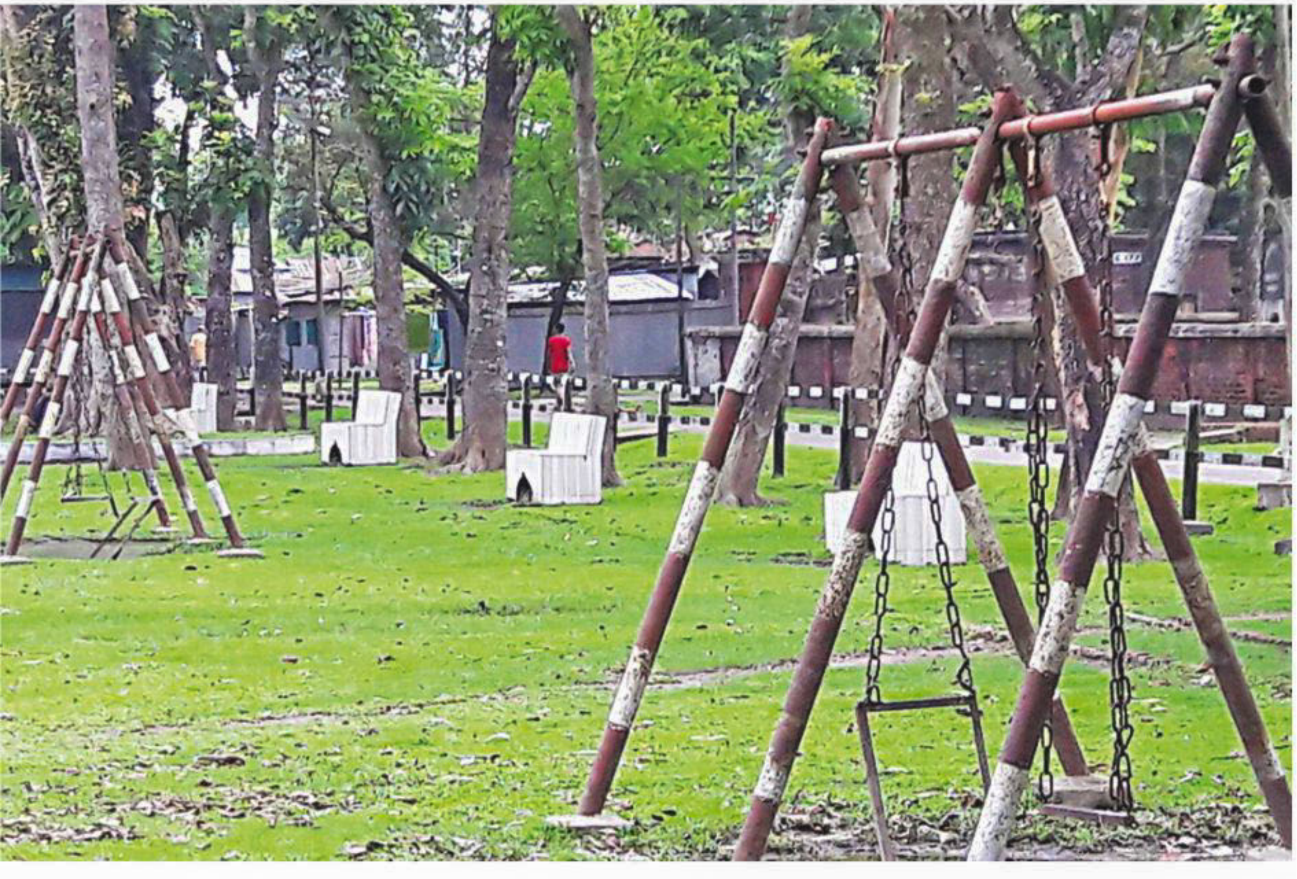
Playing equipment at railway children's park in Lalmonirhat town are damaged due to lack of maintenance.
