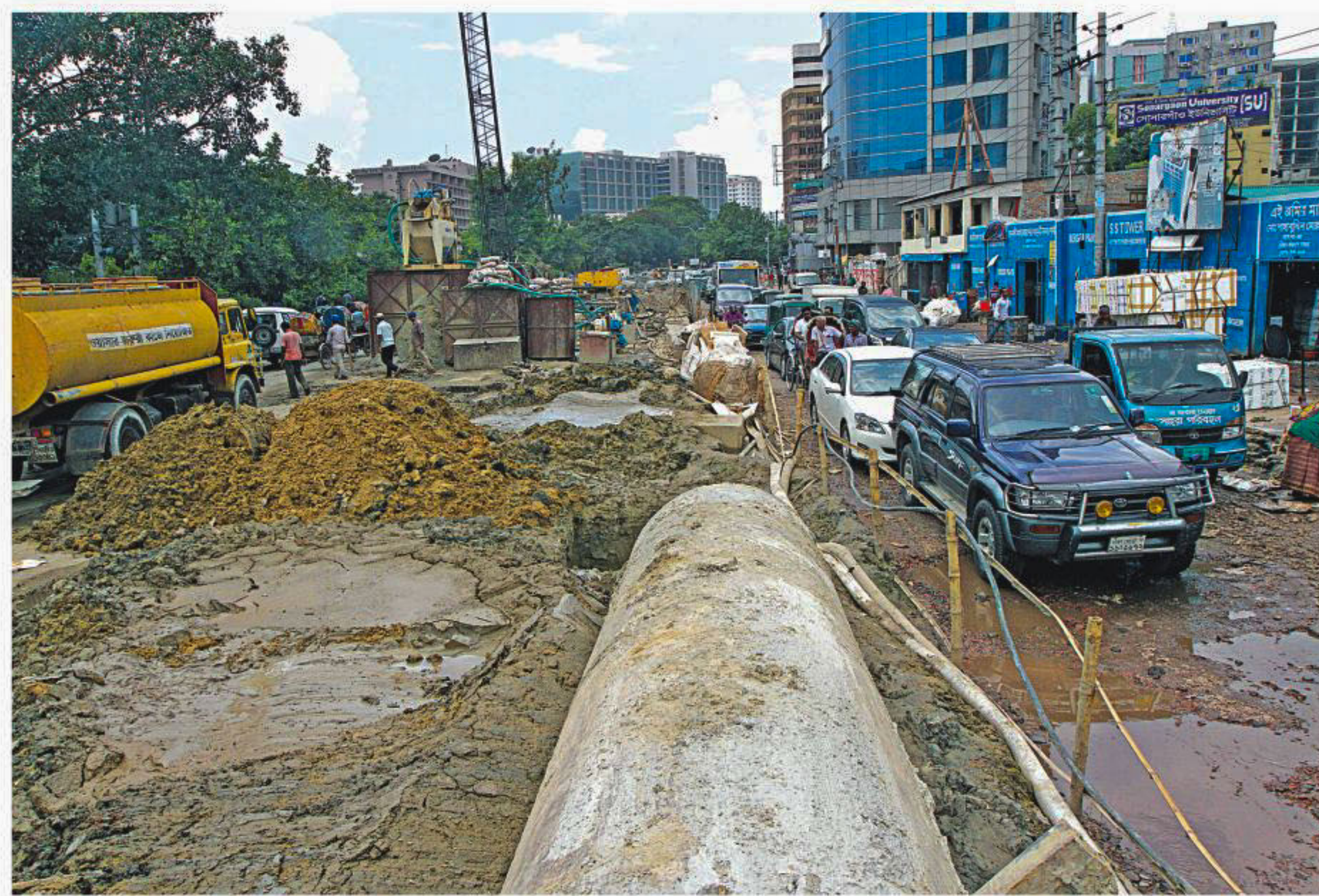
A portion of the road from the Sonargaon Hotel intersection to Hatirjheel is in an appalling state due to construction work of a ramp for the Moghbazar-Mouchak flyover in the capital. Constant digging and untidily kept construction materials have narrowed the road, making it very difficult for vehicles to cross it. The photos were taken yesterday.
