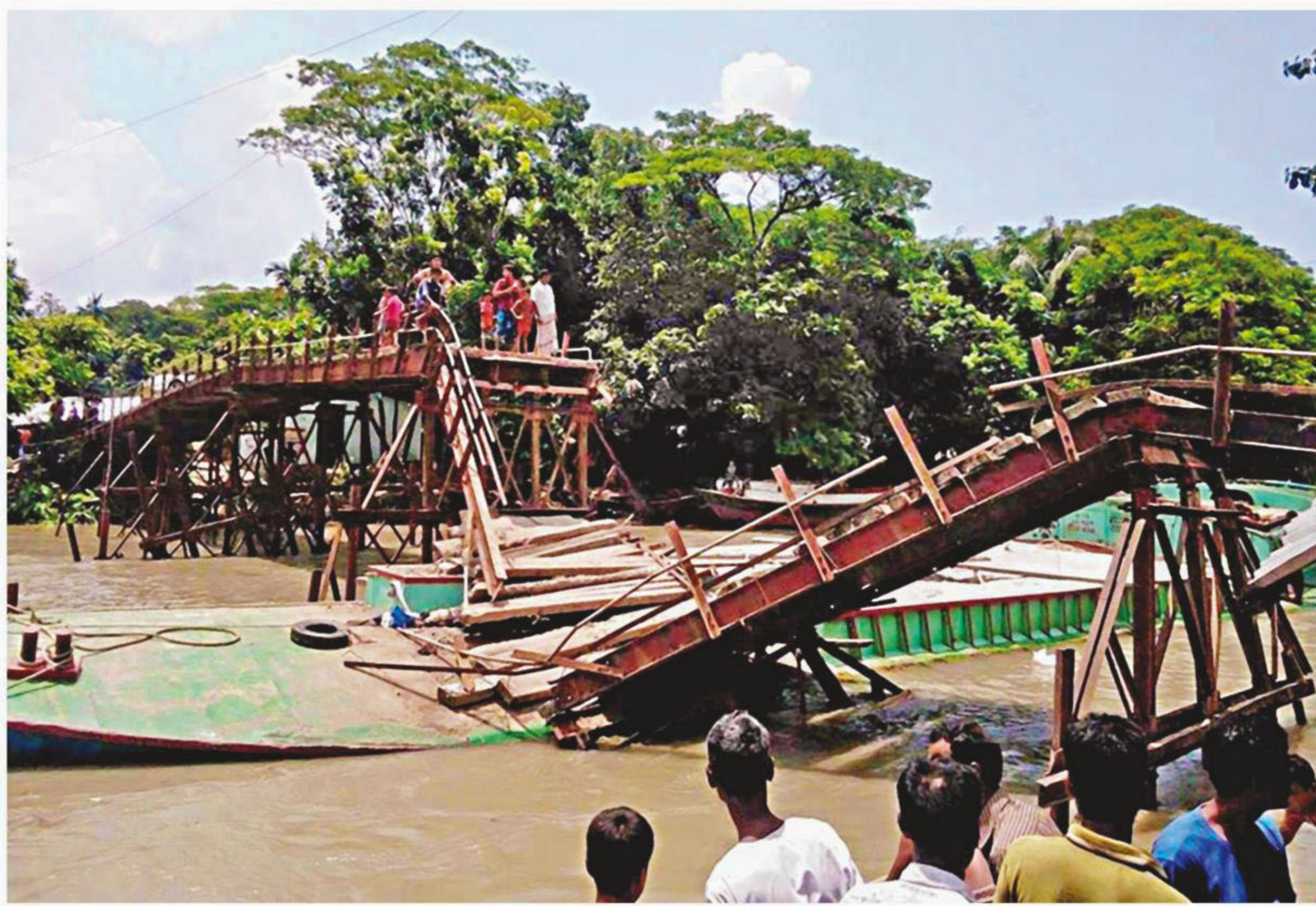
A portion of a bridge collapses on a sand-laden vessel after the vessel hit the bridge over a canal in Kalaskathi of Barisal on Friday severing road communication. The photo was taken yesterday.
