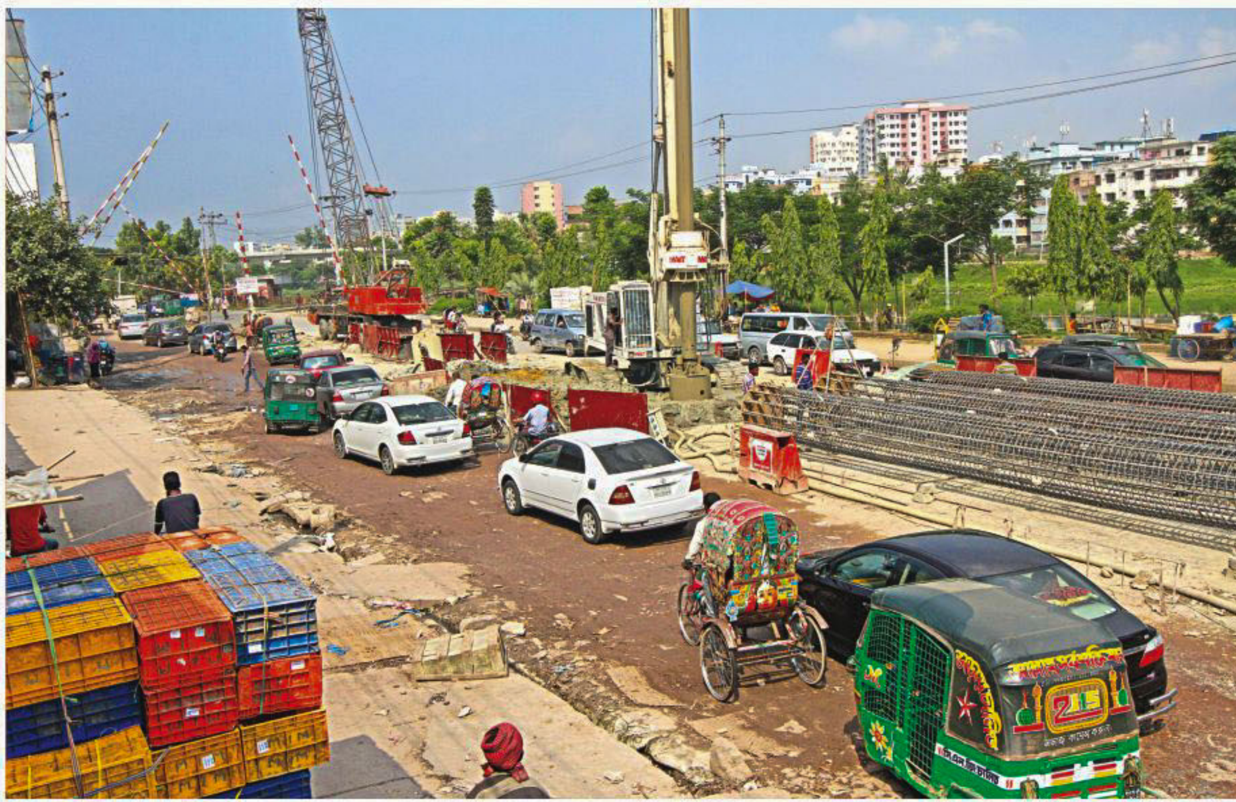
An extended ramp for the capital's Moghbazar-Mouchak flyover being built near the FDC level crossing yesterday. Experts believe the ramp could narrow down the street further and be of little use for city dwellers. PHOTO: SK ENAMUL HAQ
