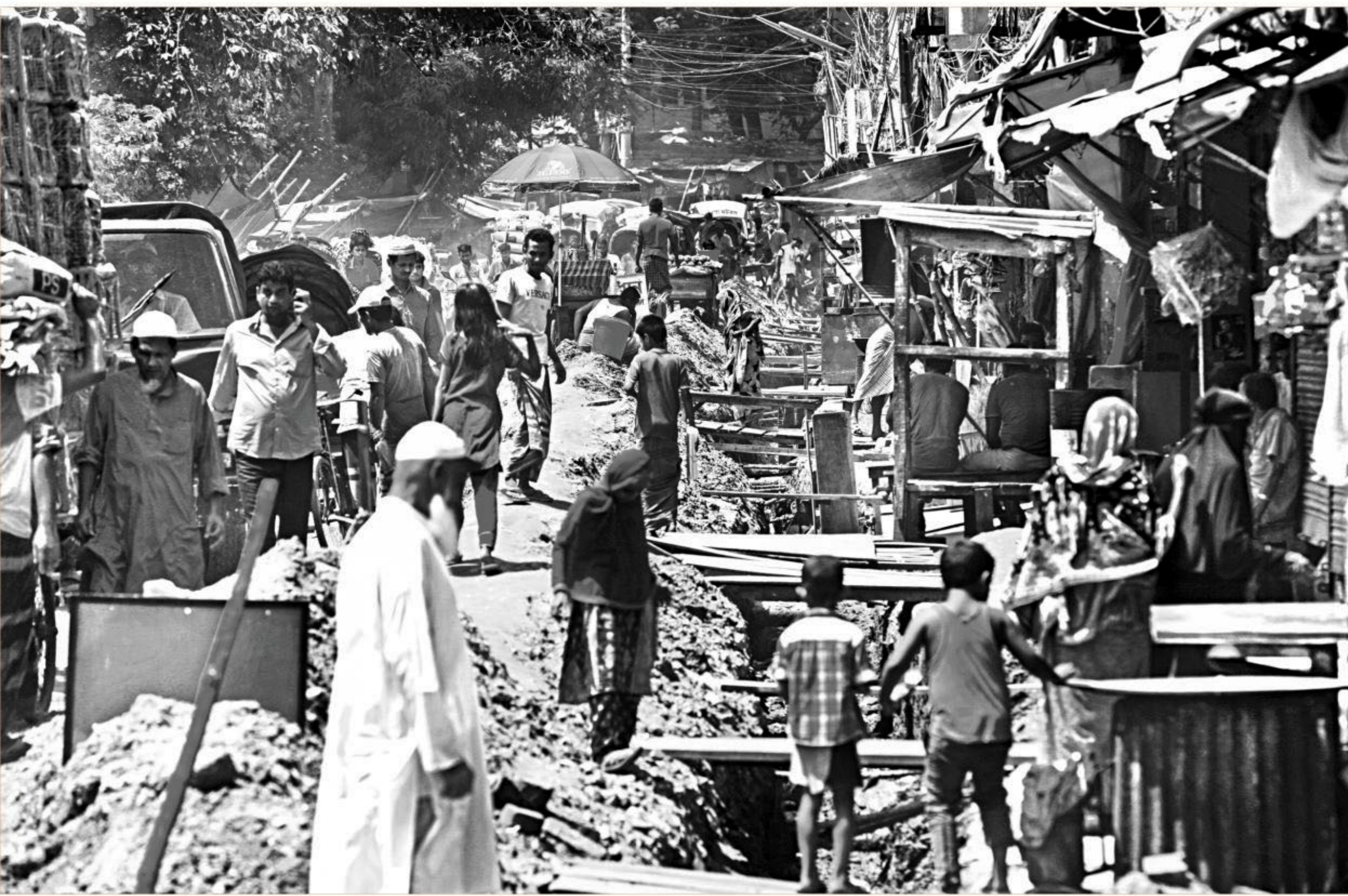
Making the life of locals and pedestrians a misery, authorities have been digging trench on a road in the capital's Islambagh for underground power cables. The photo was taken on Thursday.
