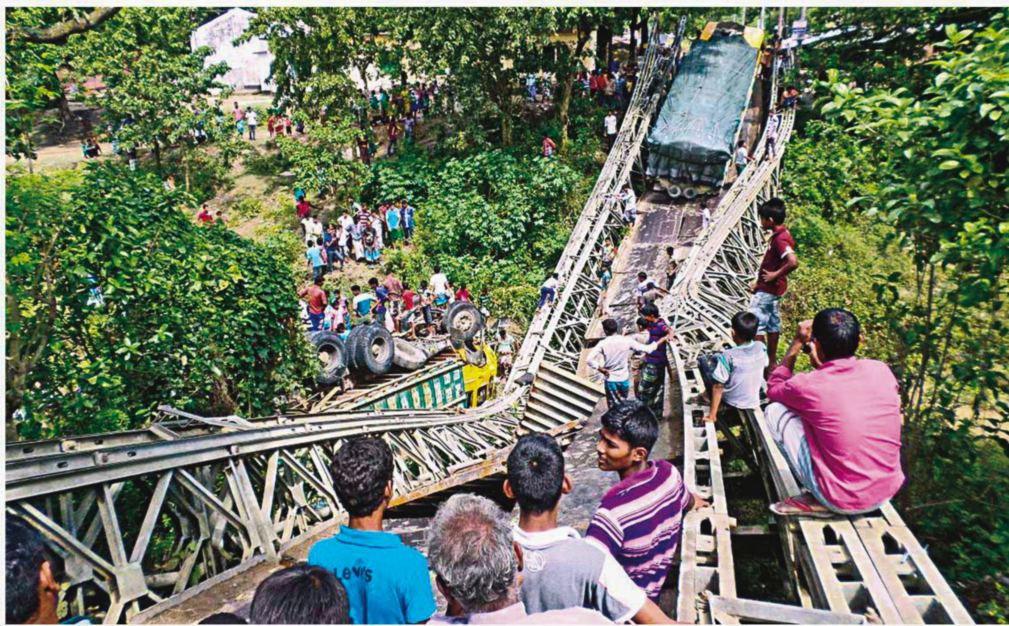
This Bailey bridge imploded due to the weight of two heavily loaded lorries on Bijoy Nagar Matikata Link Road in Rajshahi early yesterday. Two people in the truck that ended up upside down were injured.
