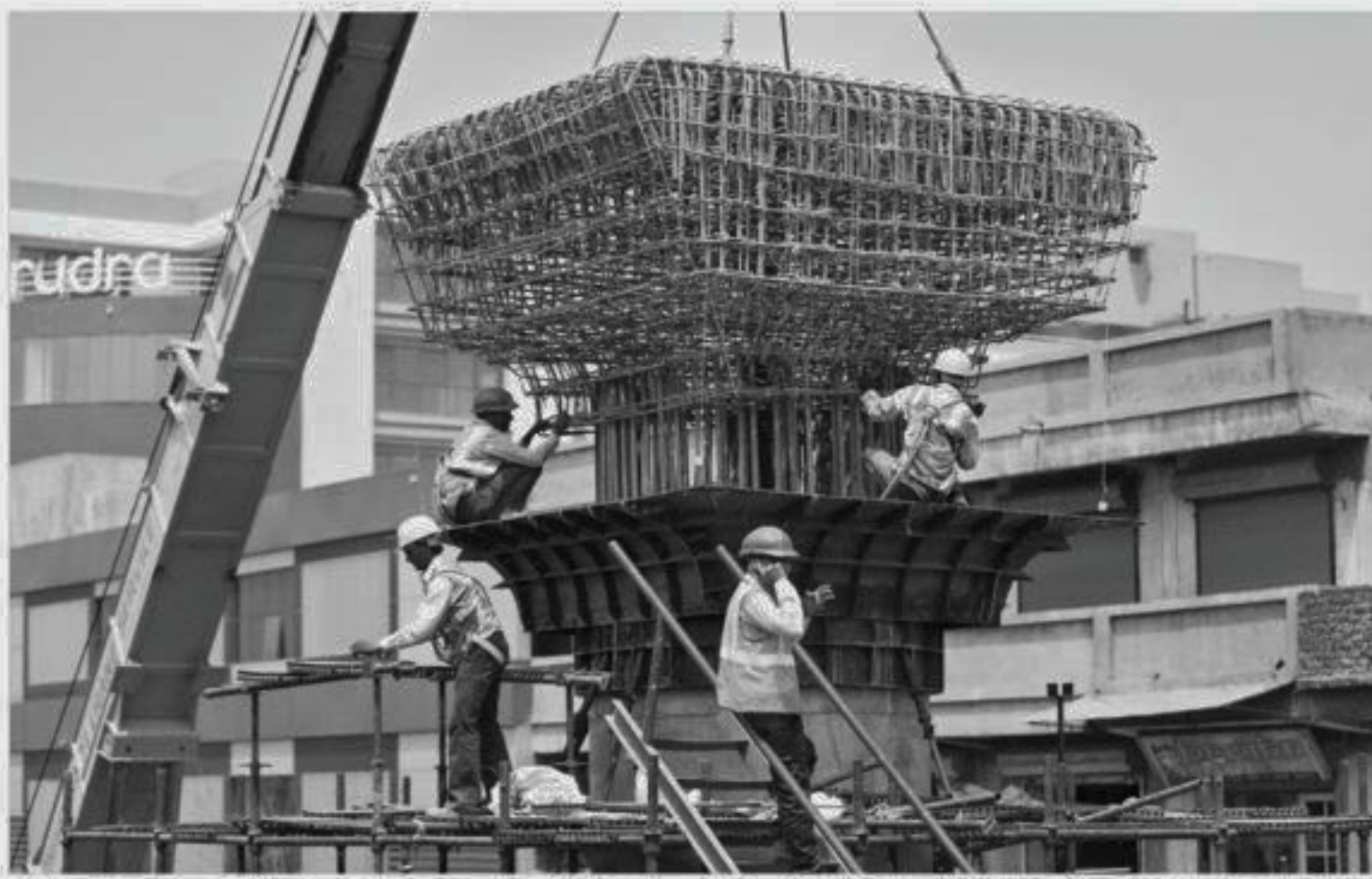
Labourers work at the site of a metro railway flyover under construction in Ahmedabad, India.
