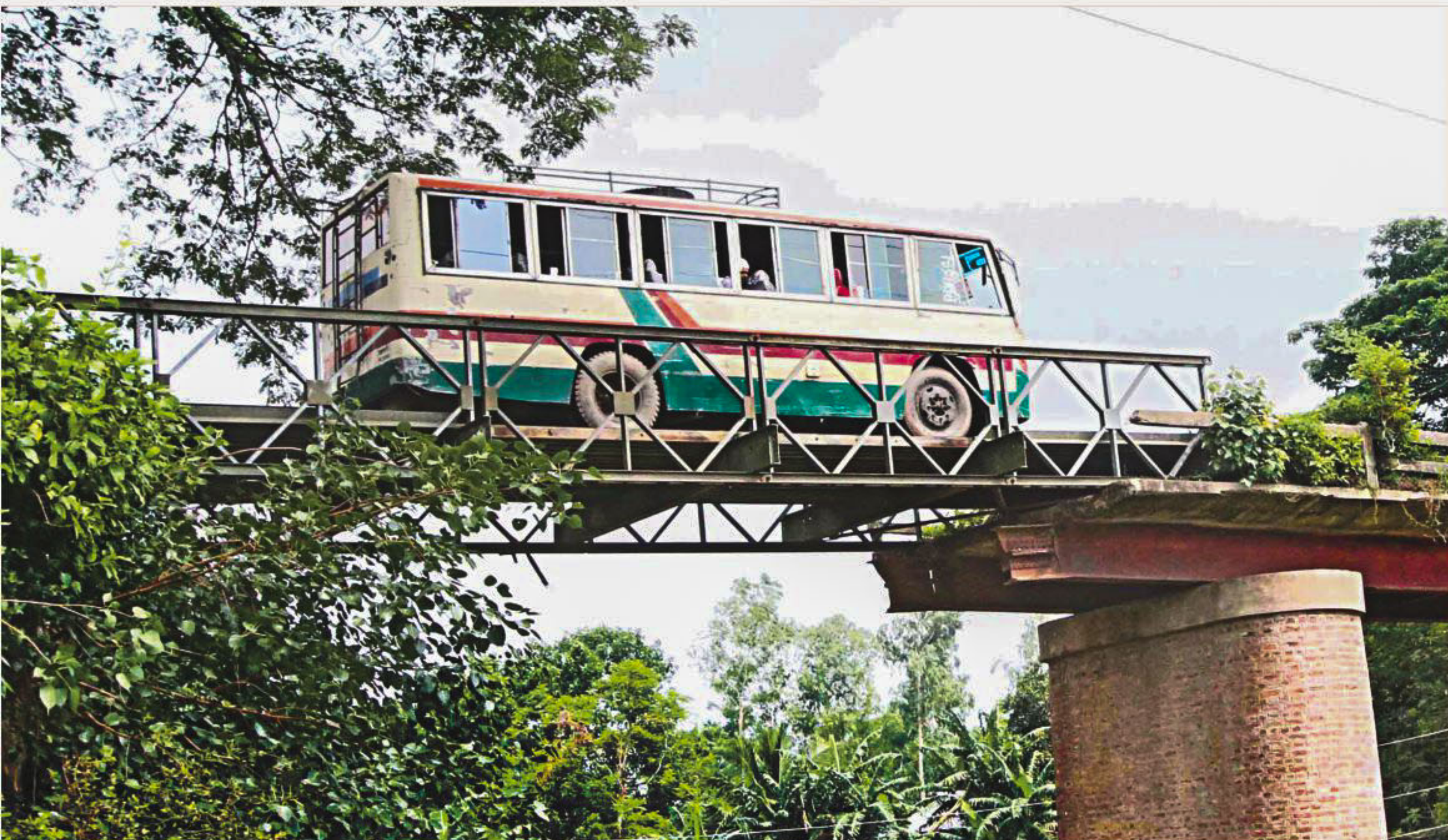
A bus goes over the precarious Rajbari Bridge on Tangail-Bhuapur Road. The bridge makes banging and squeaking noise as the bus passes. Half of it is the remnant of an old bridge built before the independence of Bangladesh and the other half is a Bailey bridge built later. The authorities concerned said a project proposal to rebuild the bridge was pending with the Planning Commission. The photo was taken on Monday. PHOTO: MIRZA SHAKIL
