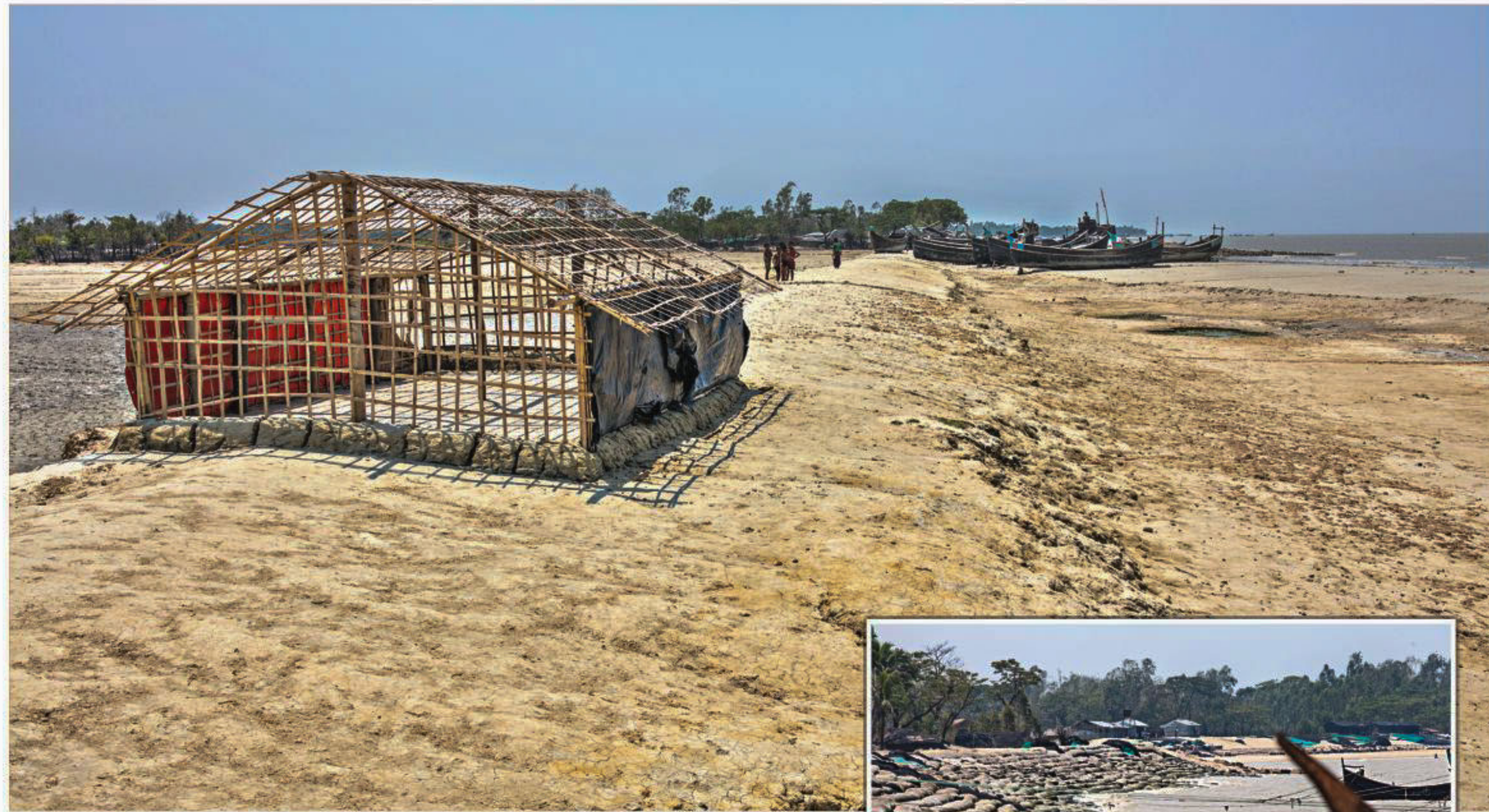
A makeshift structure under construction on a dam at Char Dhurun at Kutubdia in Cox's Bazar. The dam in this intertidal zone is in a very bad shape and that's why local fishermen, who are displaced during high tides, make homes like this. Inset, the other end of the dam protecting the offshore area. The photos were taken a couple of months back.
