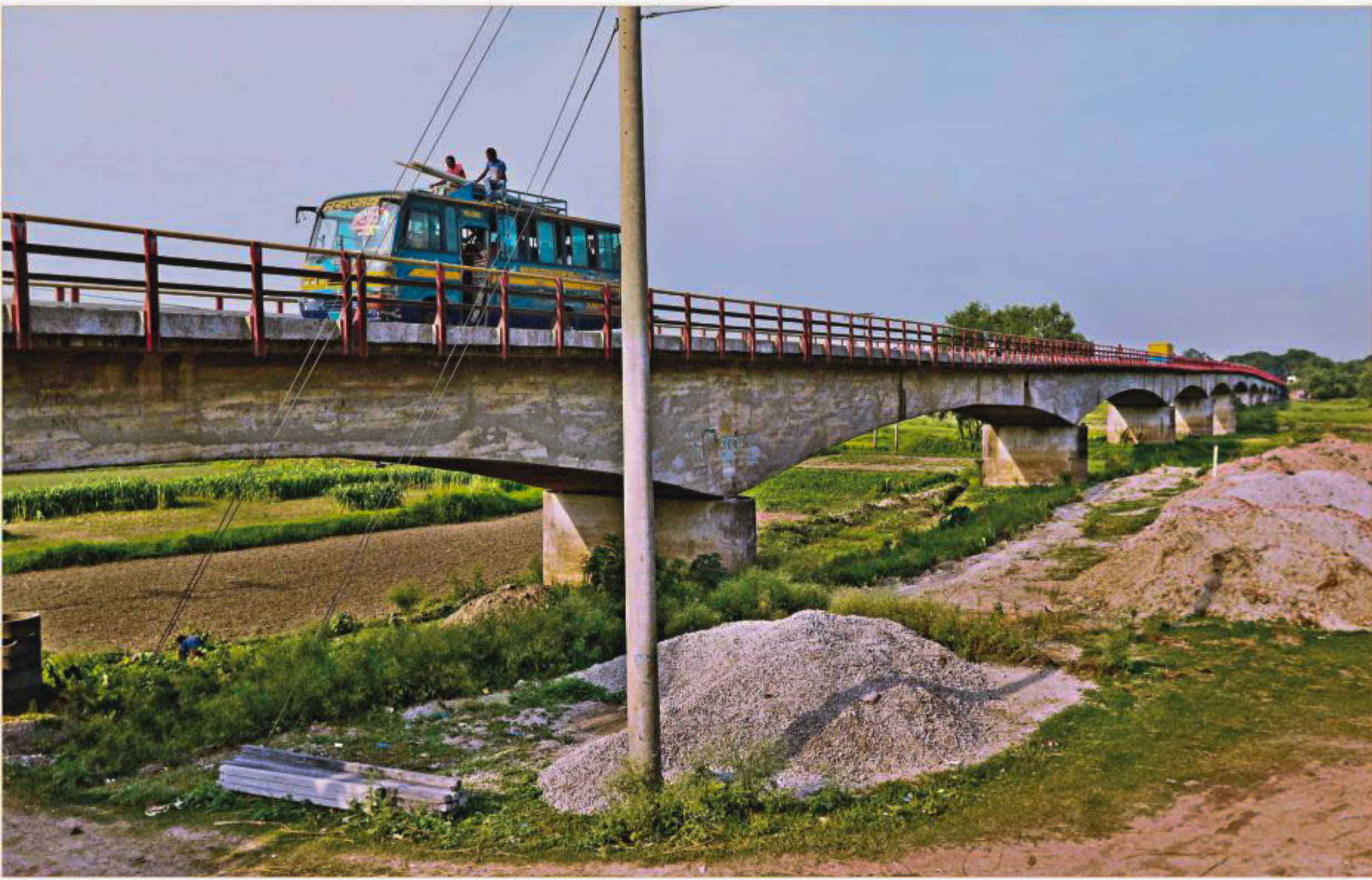
DHALESHWARI IN DANGER: This huge bridge over the Dhaleshwari river in Jagir area of Manikganj sadar is evident how mighty once the river had been. Sadly today, it is absolutely dry at places like this, as silt accumulated and blocked the water flow in nearby Tittli area. Locals have long been demanding urgent steps to save the river in vain. The photo was taken last week.
