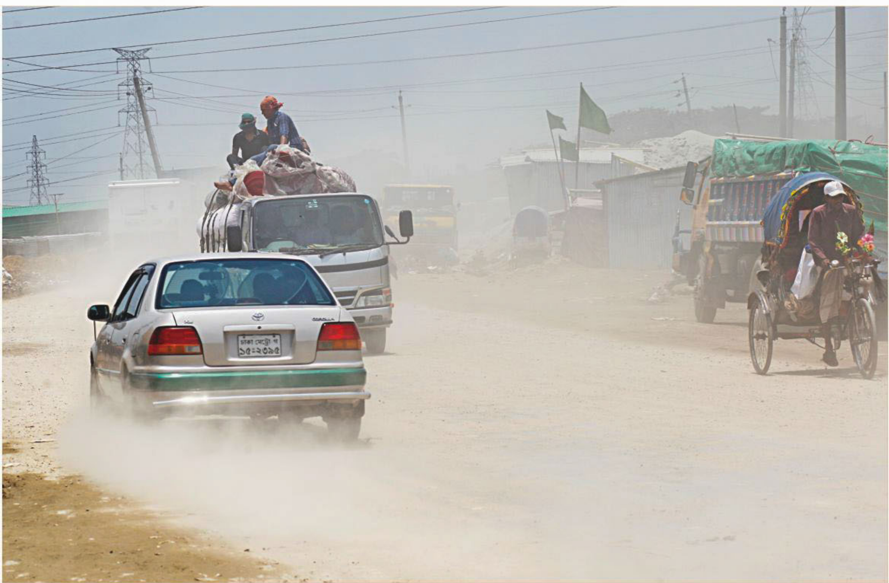
Dust cloud makes journeys hellish on the heavily battered Gabtoli-Babubazar Beribadh (embankment road), on the western edge of the capital. It also creates a huge possibility of accidents. The photo was taken on Thursday at the Gabtoli end.
