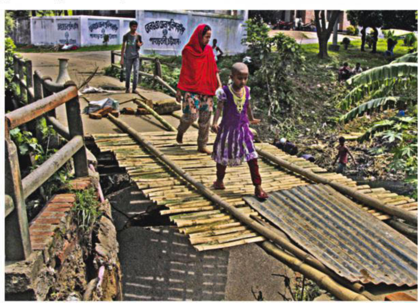
This culvert in Pahartoli Railway Police Line area of the port city fell apart hit by cyclone Roanu. PHOTO: ANURUP KANTI DAS
