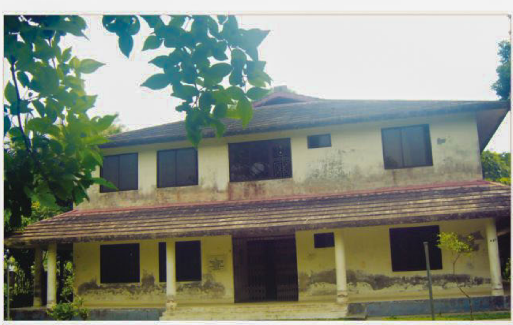
Nazrul Memorial Centre in a derelict condition. PHOTO: STAR
