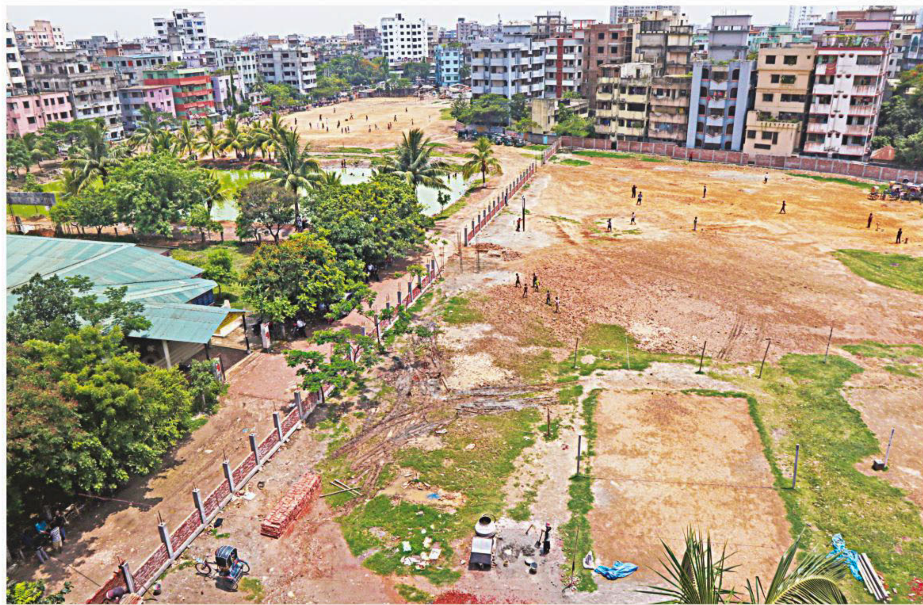
Basabo Balurmath in the capital is under a severe threat as the government has already started constructing a boundary wall to turn a portion of the field into a school and a college, depriving the citizens of the joy of an open space. The photo was taken yesterday. PHOTO: AMRAN HOSSAIN
