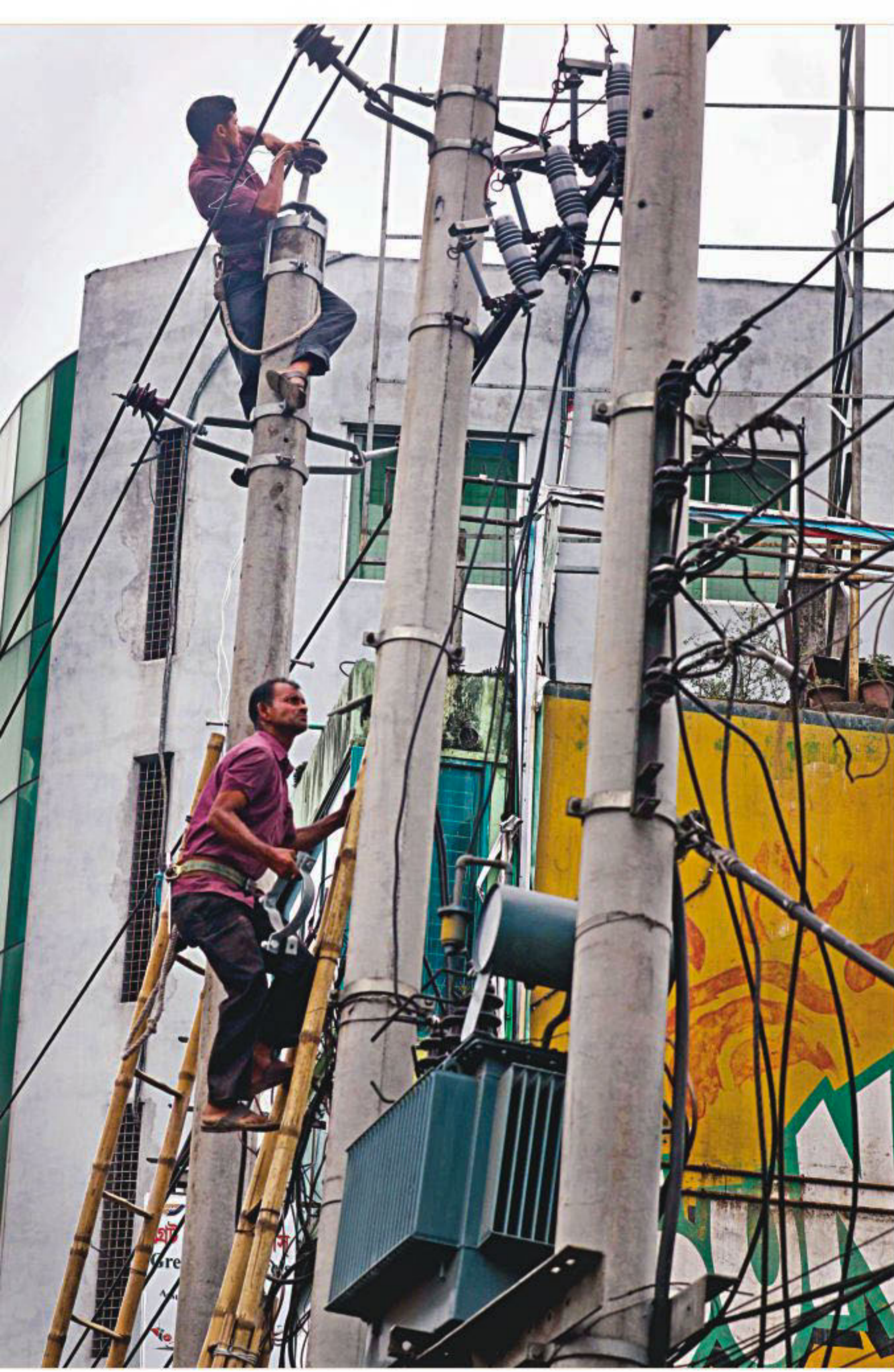
Without wearing enough protection gears, two men work on a high-voltage transformer installation on Kazi Nazrul Islam Avenue in the capital yesterday. Electricians often die from electrocution in such circumstances but their safety issue remains unaddressed. PHOTO: PRABIR DAS
