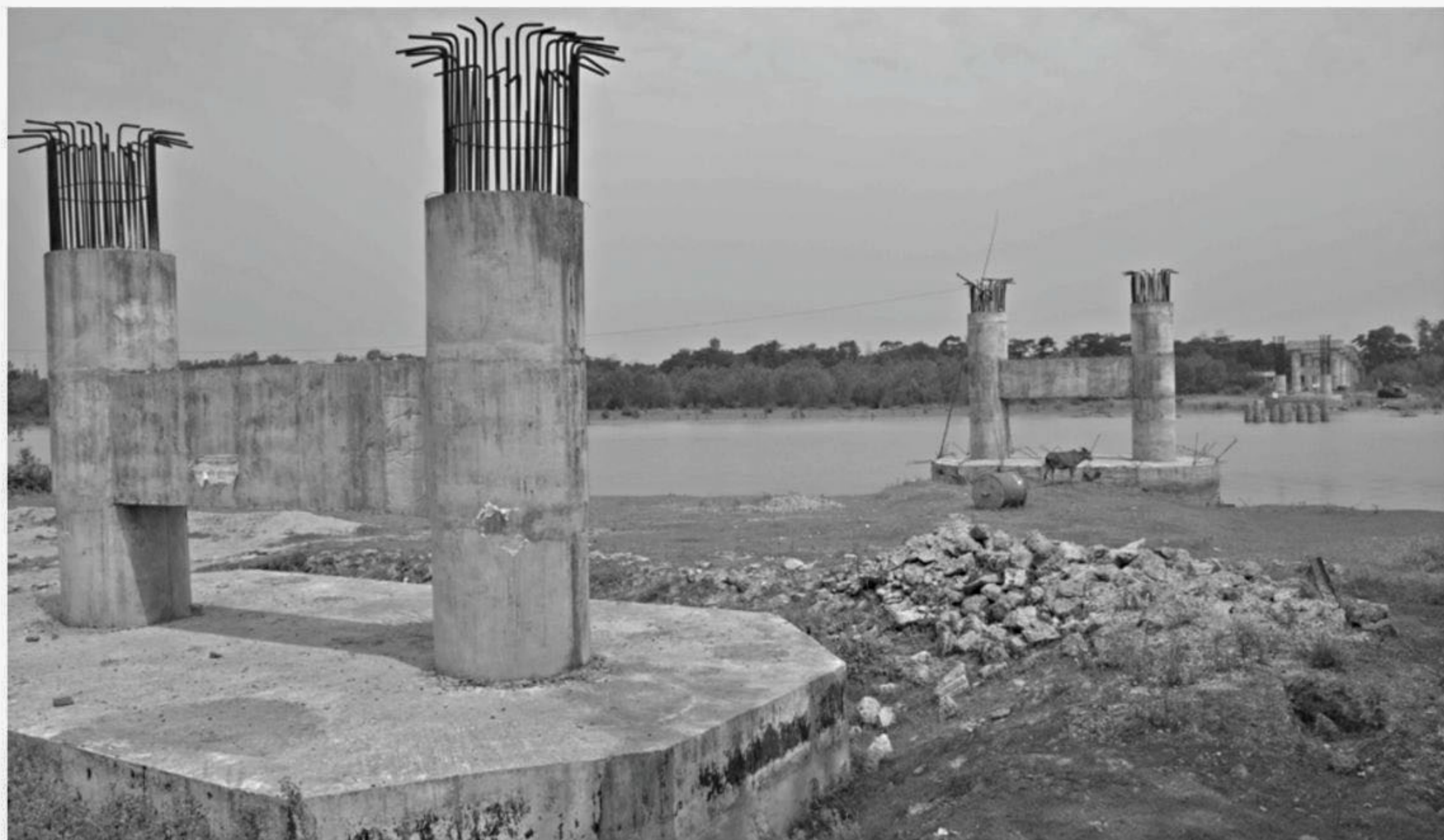
Construction work of Lohalia Bridge on the Lohalia River on Patuakhali-Dashmina road remains suspended for over a year.
