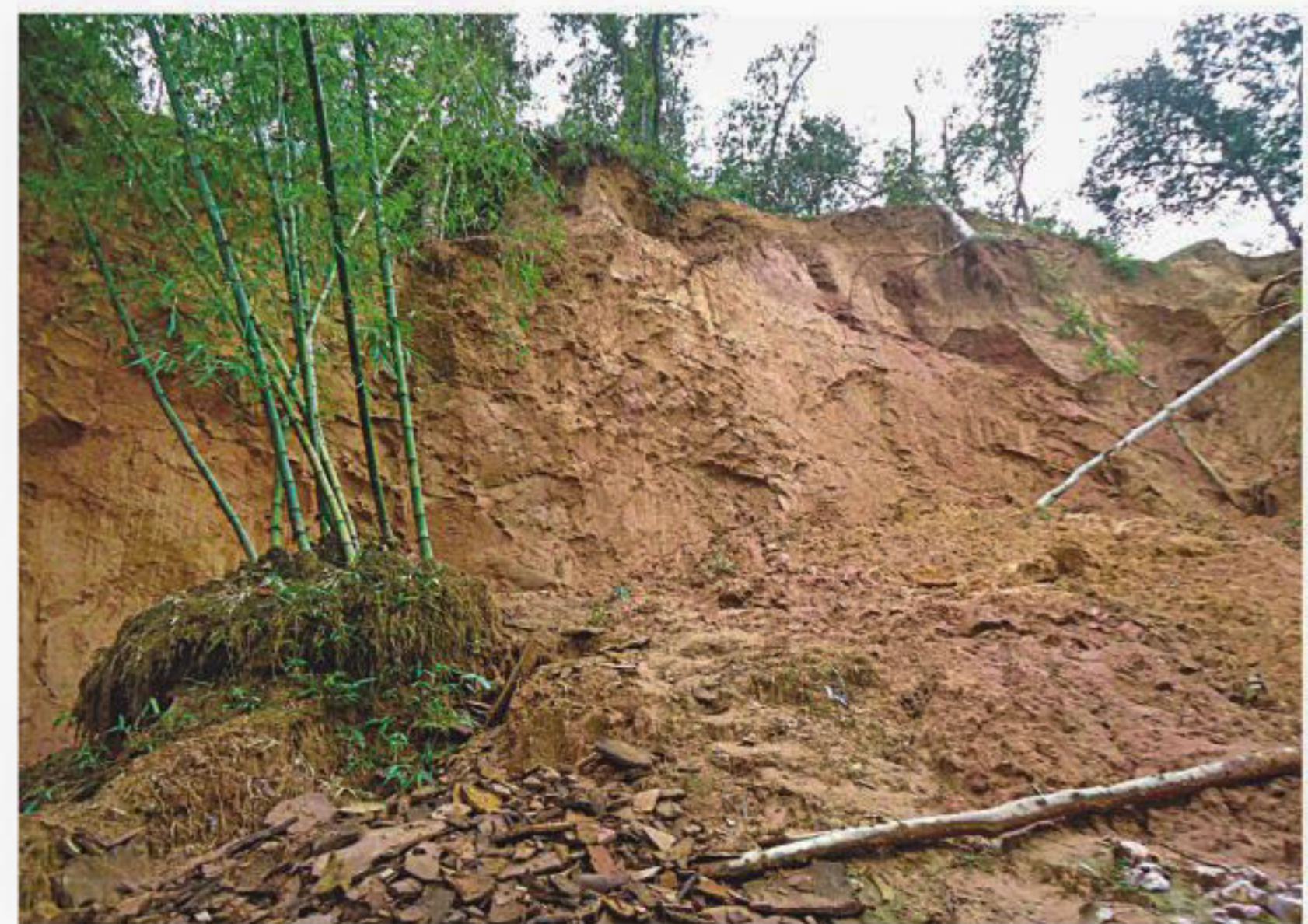
A hillock in Montoil village of Juri upazila in Moulvibazar. Several dozens of families in the village are passing their days in fear of landslides due to a flood triggered by rain and the onrush of water from the upstream. The photo was taken recently. PHOTO: STAR
