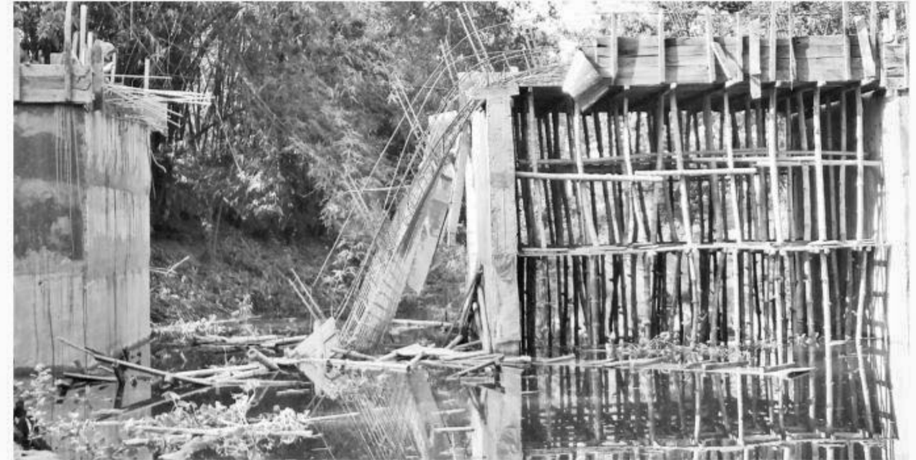
An under-construction bridge collapsed, injuring four workers, at Jolarkandi of Natore Sadar upazila yesterday noon, apparently due to serious fault in the construction work.
