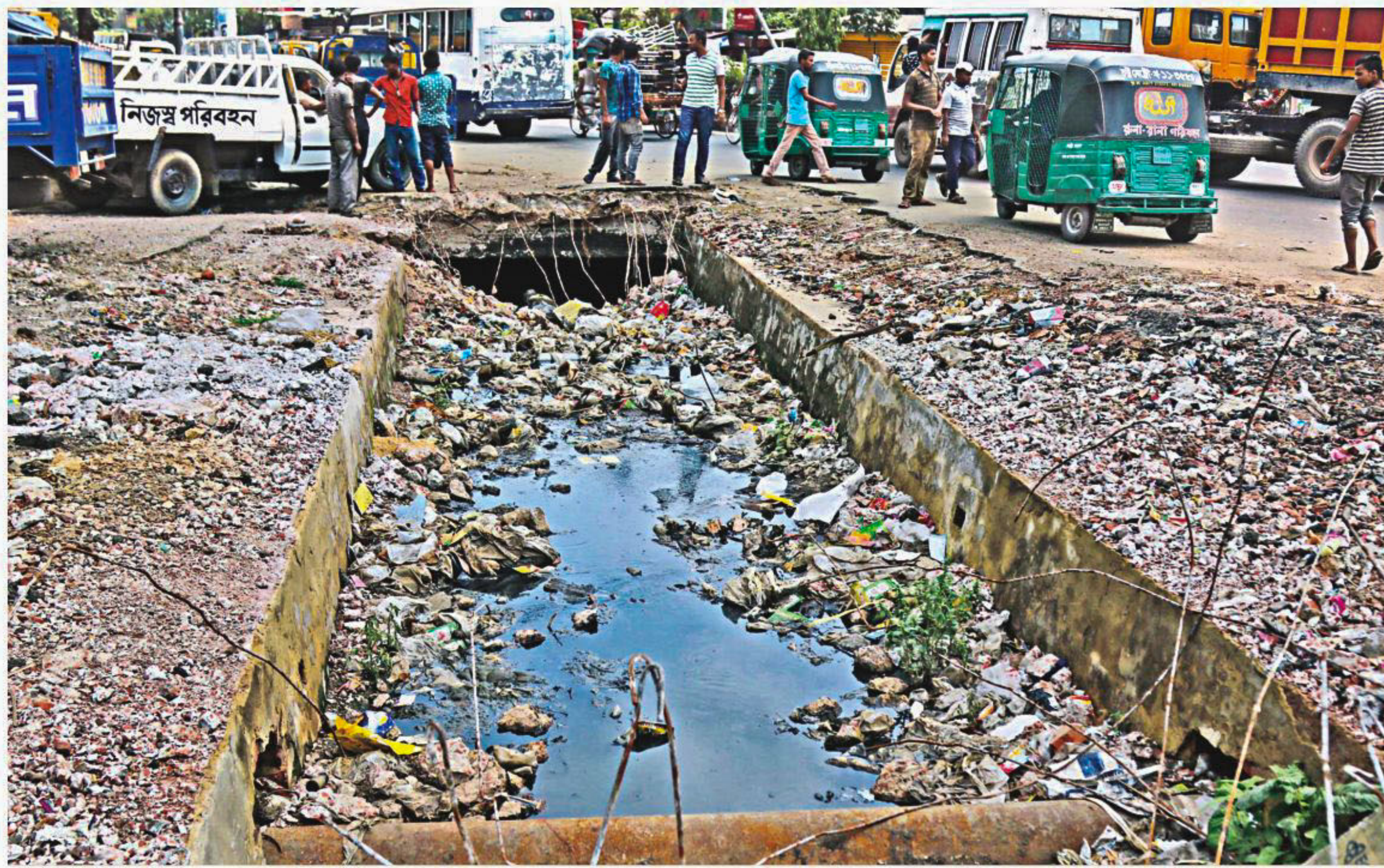
The Chittagong City Corporation removed the concrete cover over this drainage outlet right underneath the busy road at Sagarika intersection after an explosion, caused by trapped gas, blew off part of the slab on February 10. Though the breaking of the slab was done to check the possibility of further explosions as an immediate precautionary measure, the authorities have not constructed a new cover since then, seriously hampering vehicular movement in the area. The photo was taken yesterday.
