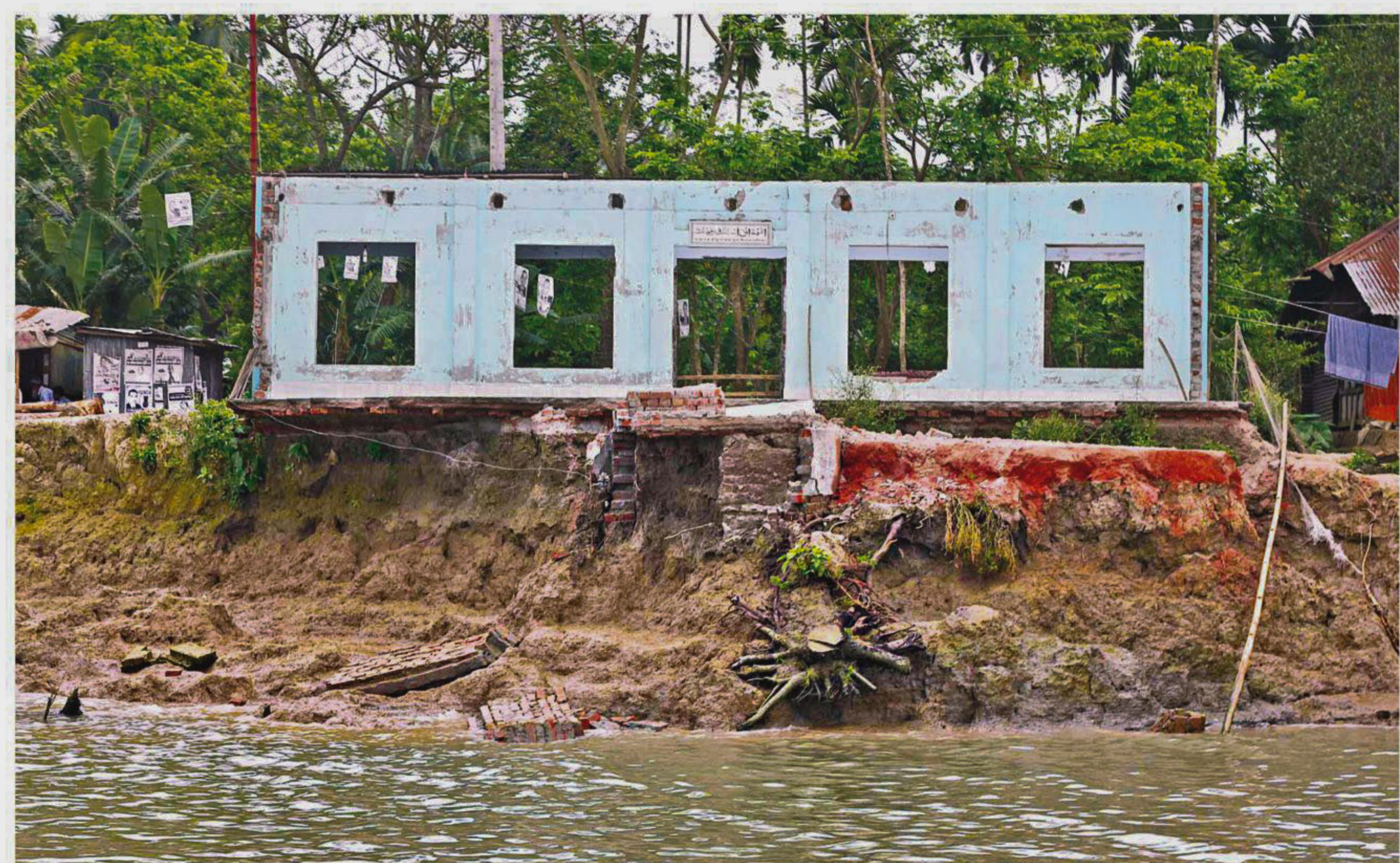
These remains of a building in Janata Bazar of Barisal yesterday, used to be a mosque, which was the only one in the area. It also is not the only structure that got and is getting devoured by the Kirtankhola River, owing to onrush of water for the last couple of days from the upstream during the high tide, over a long stretch including the areas of Charbaria, Beltola, and Charkaua Kheyaghat as well, rendering hundreds homeless.
